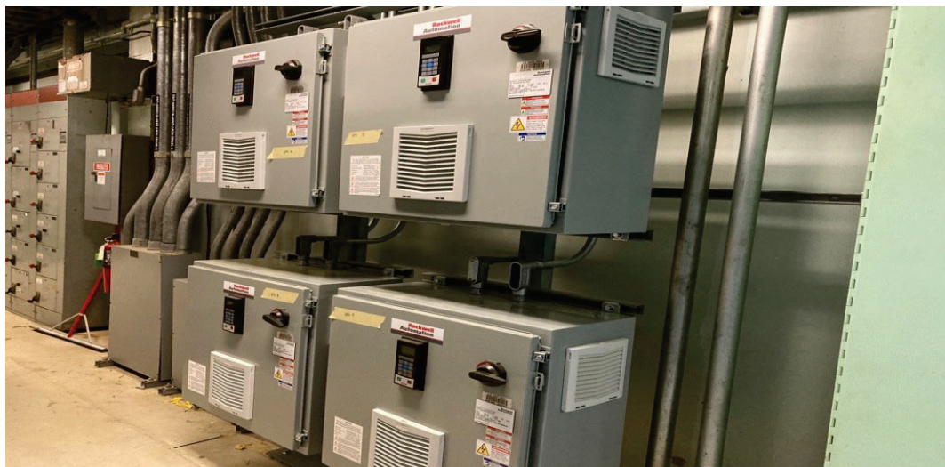
Figure 15: Tank 39H Turntables VFDs
