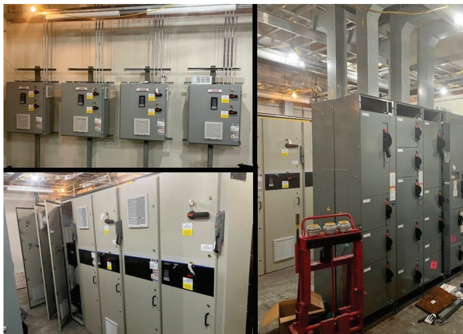
Figure 8: New Electrical Control Room Motor Control Centers and Variable Frequency Drives
