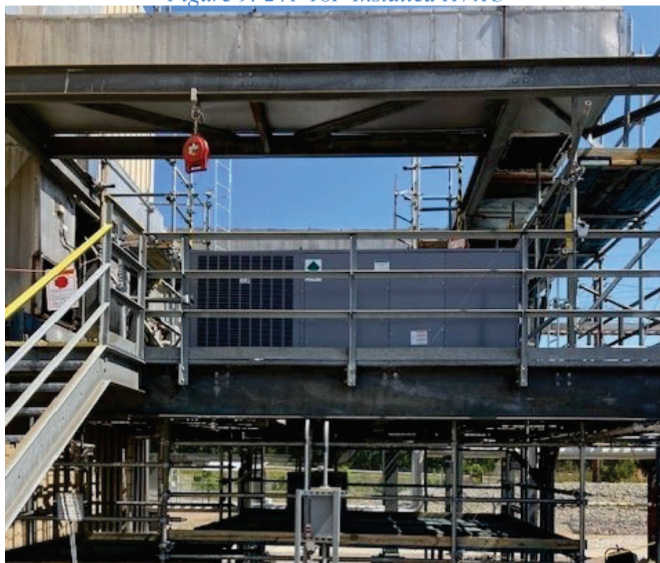
Figure 9: 241-18F Installed HVAC
