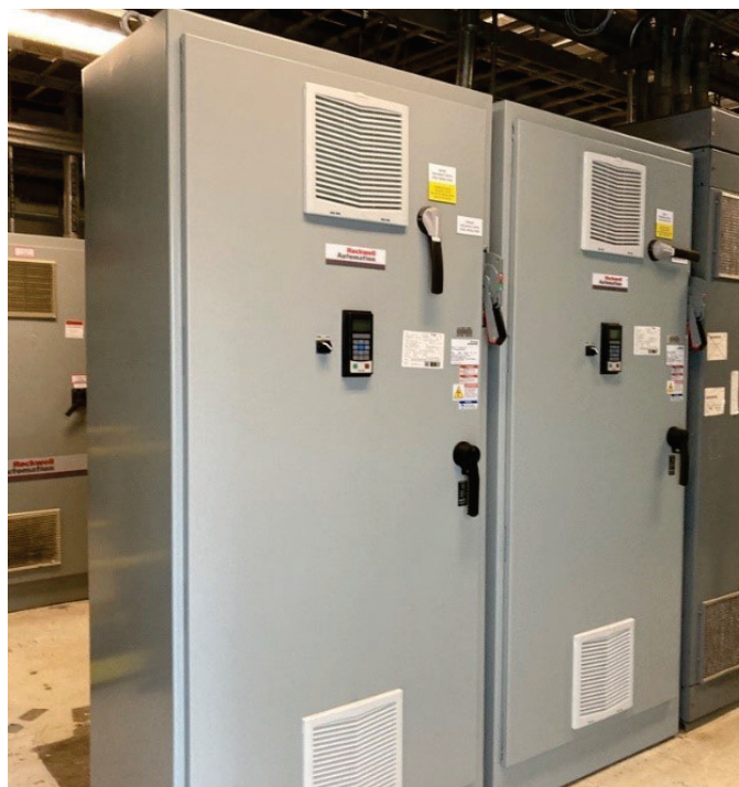
Figure 16: Tank 39H CSMPs VFDs
