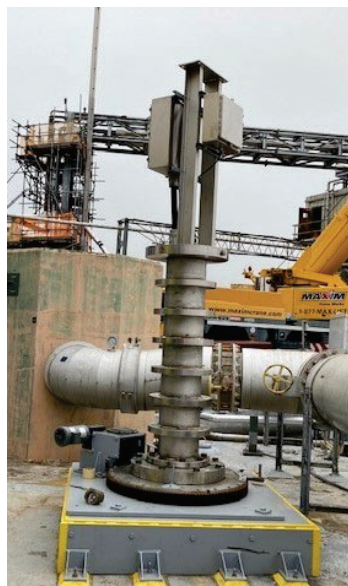
Figure 14: Tank 39H Riser B3 CSMP
