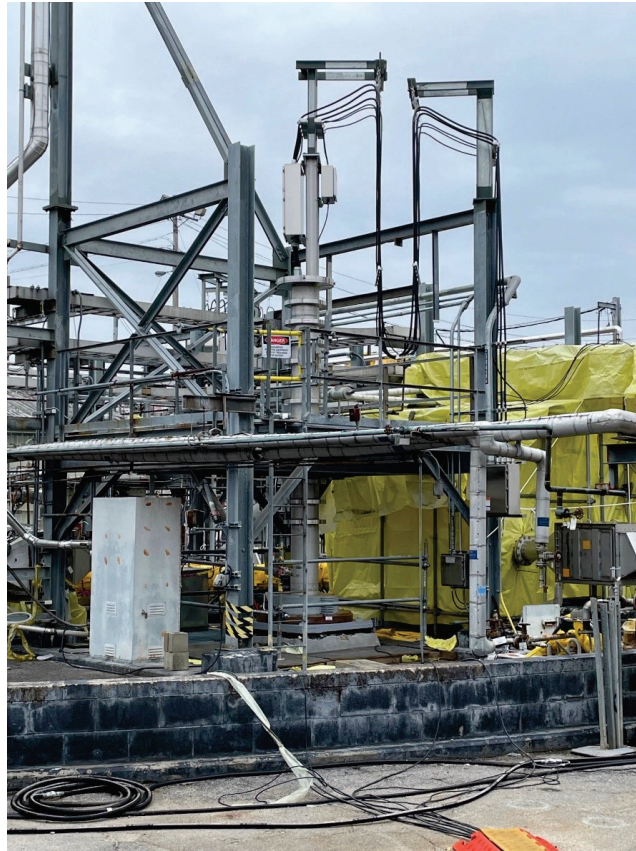
Figure 4: Tank 10 Riser 4 Commercial Submersible Mixer Pump
