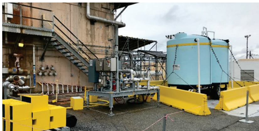
Figure 4: Tank 27F Water Addition Pump Skid
