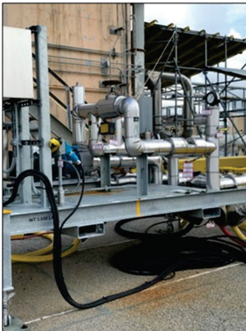
Figure 11: Tank 44F Water Addition Pump Skid Piping/Valves
