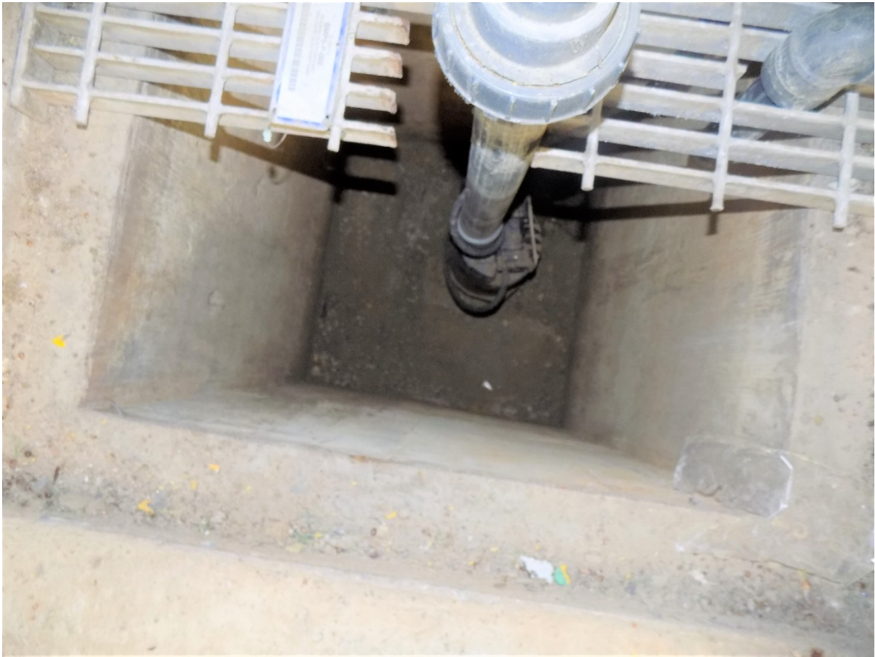
Figure 8. 607-14D Collection Sump
