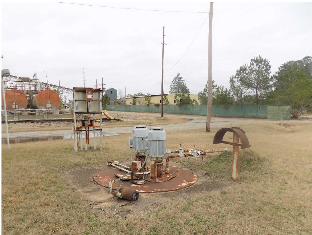
Figure 13. Sanitary Sewage Lift Station 607-12D (currently abandoned)
