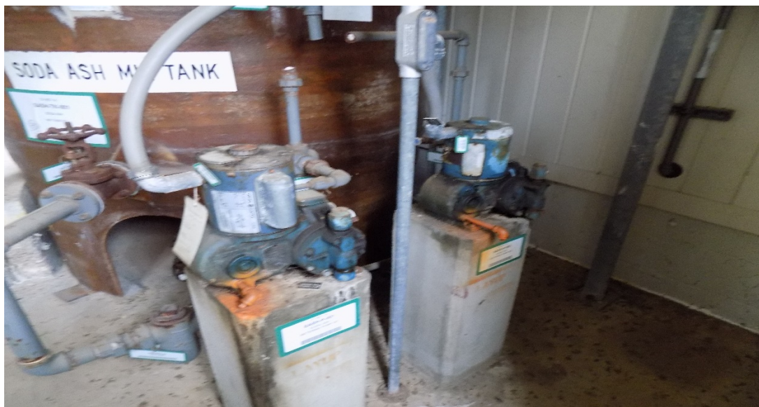
Figure 7. Soda Ash Transfer Pumps/Pedestals (607-14D)
