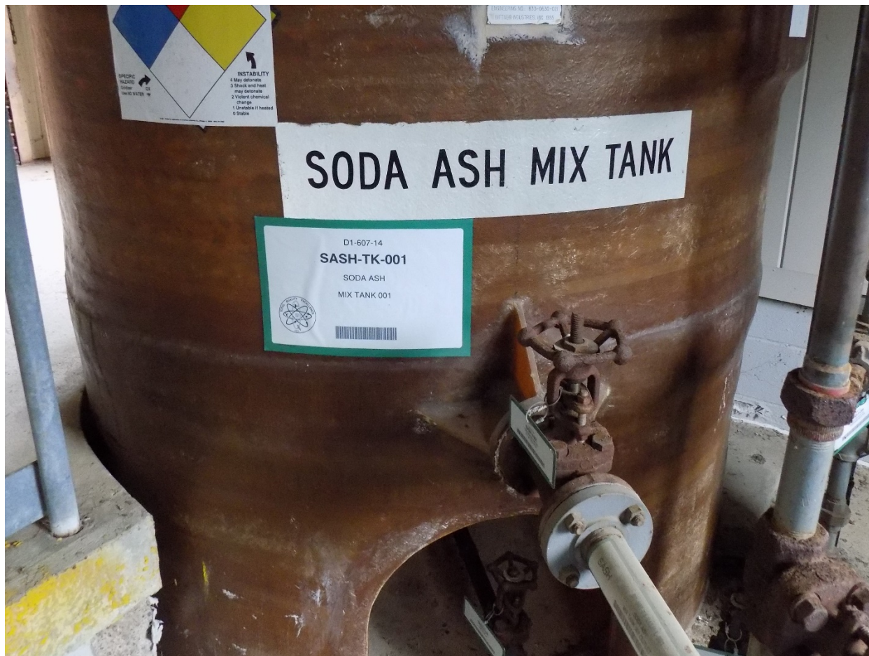
Figure 6. Soda Ash Mixing Tank (607-14D)
