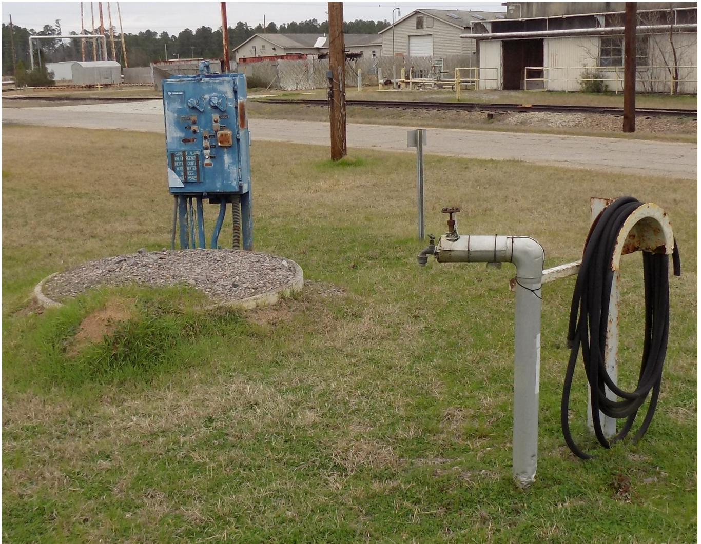
Figure 14. Building 607-2D, Sewage Lift Station #2 and Process Water Hose Connection
