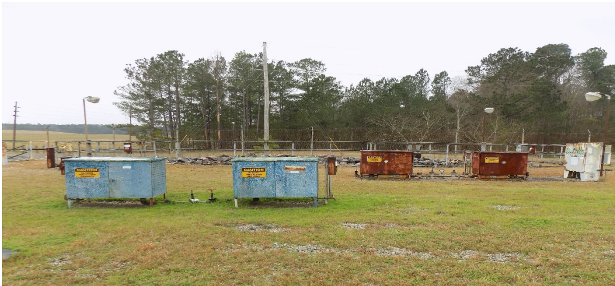
Figure 11. Building 607-15D Blowers
