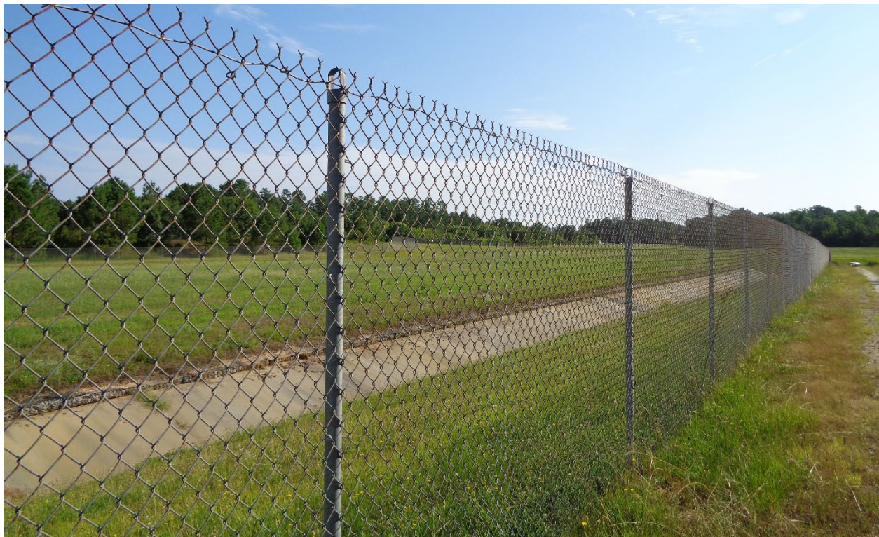
Figure G-4. Current On-Unit Photographs of the Cover System of the HHWMF OU (2020)
