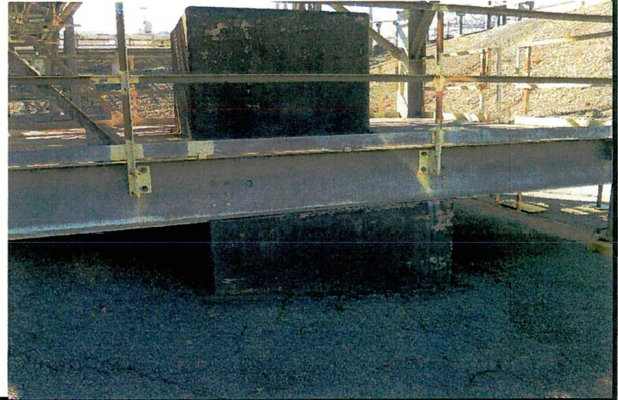
Tank 19, West Riser
