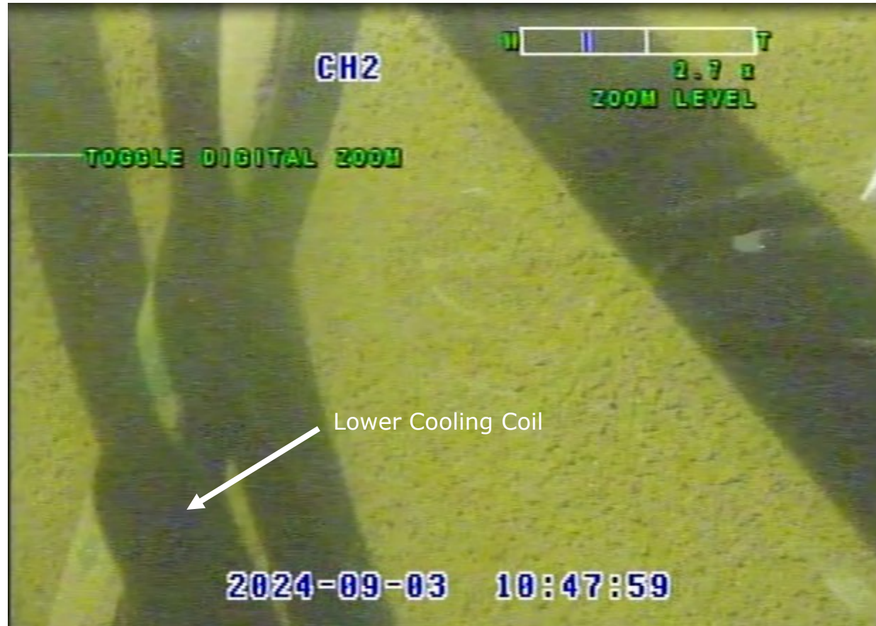
Riser 4 down towards SW quadrant floor
