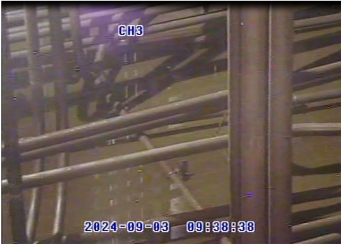
Riser 2 looking NW
