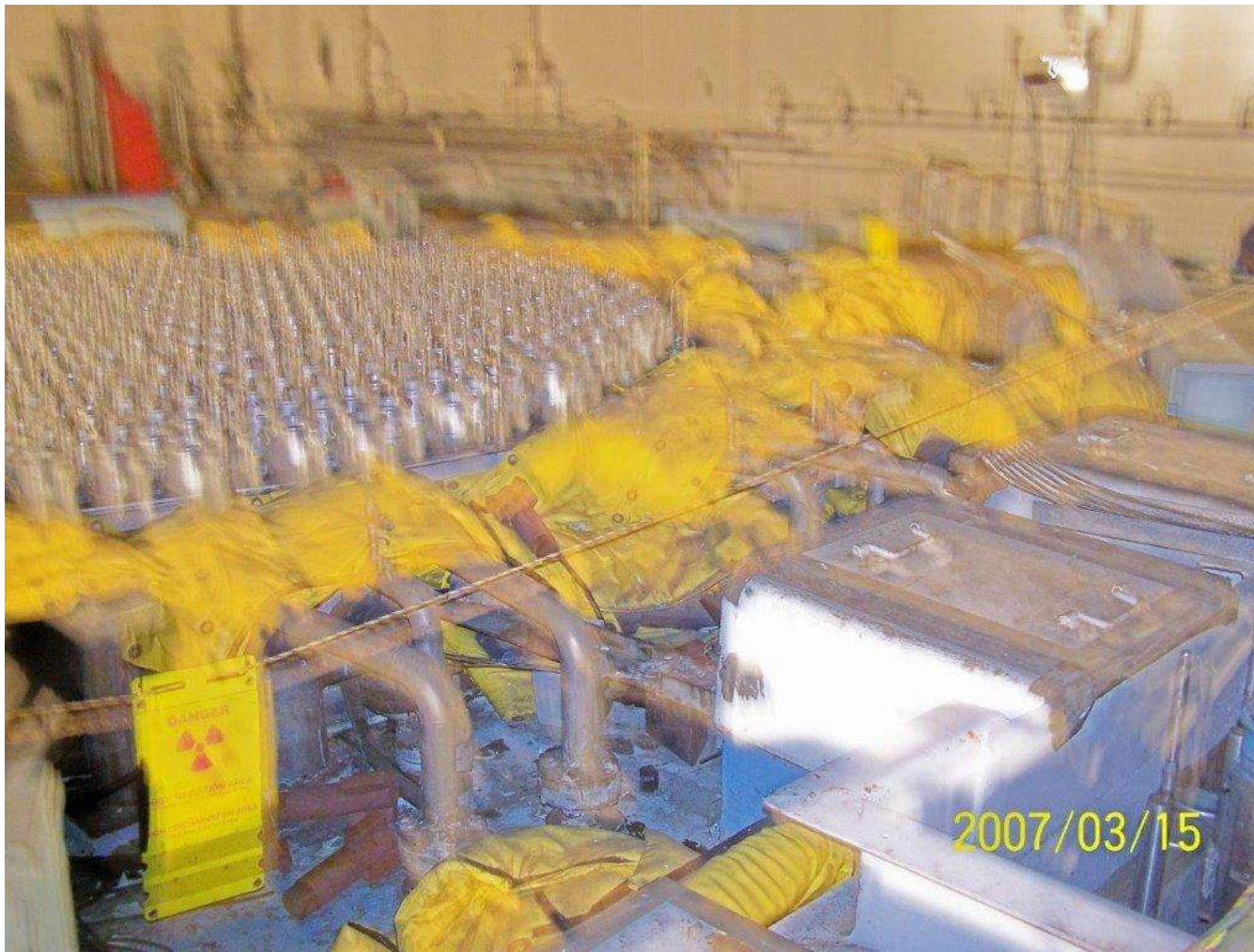
Figure 2.2 Process Area Lead in Photo Taken During Maintenance Activities in March 2007
