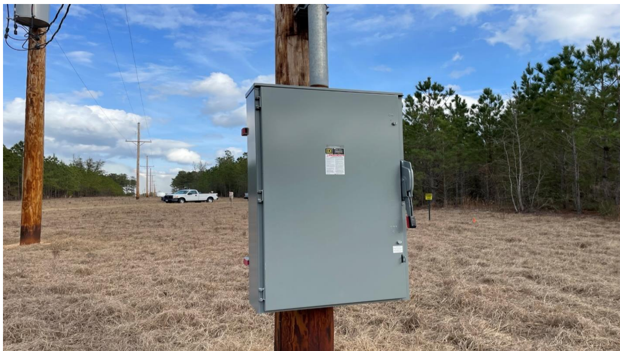
Photo 12: View of power box located on the existing utility pole.
