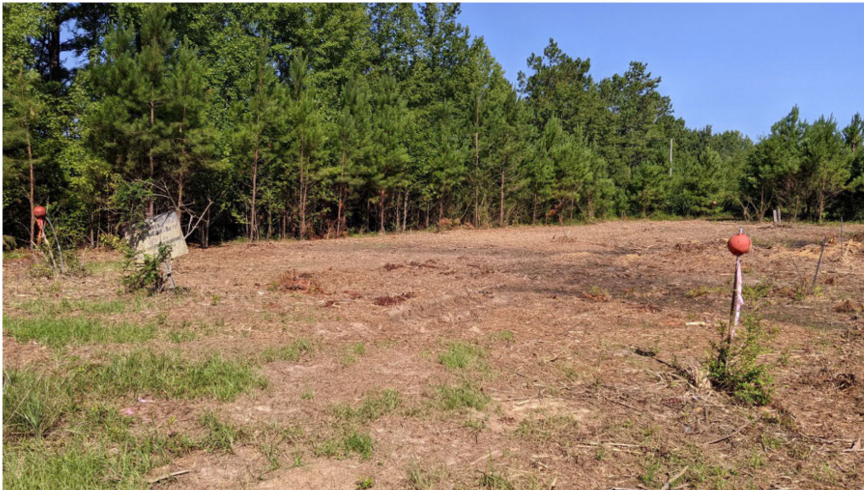
Figure 2-4. Photo of the LRP 131-1L Subunit Following Clearing to Support the RFI/RI Characterization Sampling (2022)
