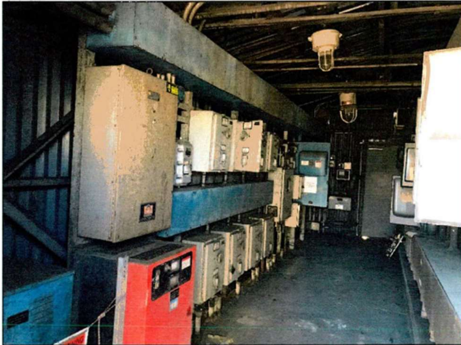
Figure 11. Inside the Coal Handling Control House
