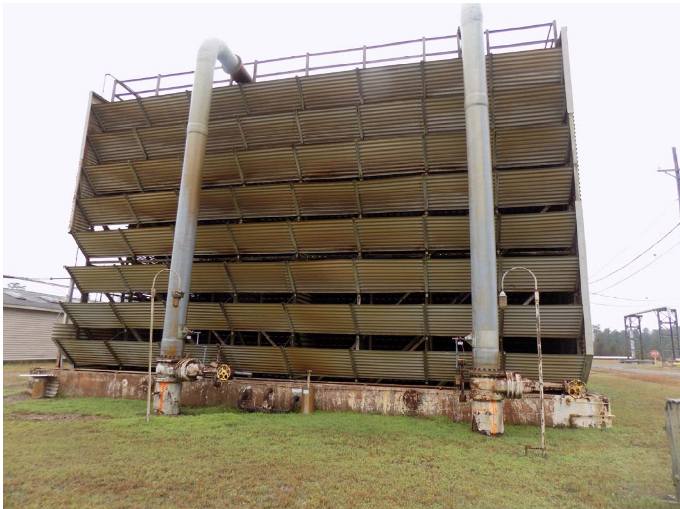
Figure 5. Building 485-D, D-Area Cooling Tower Water Return Lines
