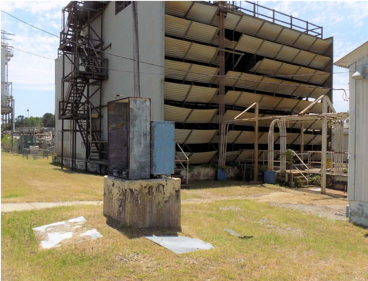
Figure 7. Building 482-2D, Outside Electrical Cabinets
