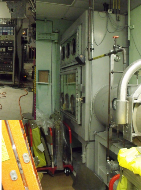
Maintenance GB, Room 1002
