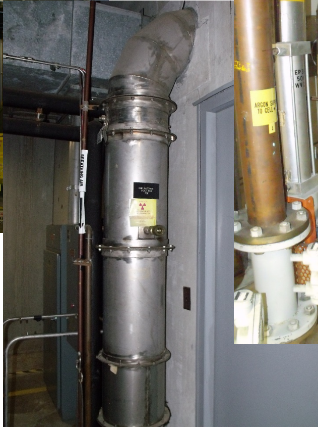
PEF Exhaust Duct, Room 234
