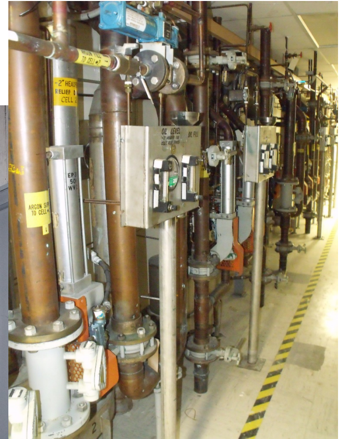
Contaminated Equipment (Piping), Room 2010
