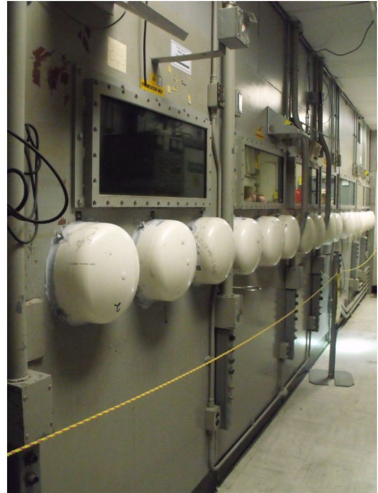
Gloveboxes 3-6, Room 154 (Operating Side)
