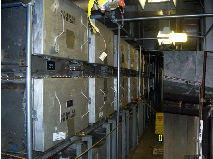
HEPA Filter Banks, Room 2000
