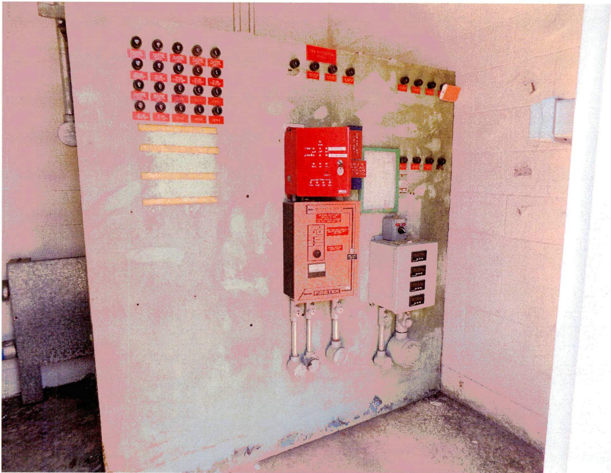
Figure 7. Fire Panel and Control Room (Looking Northeast)
