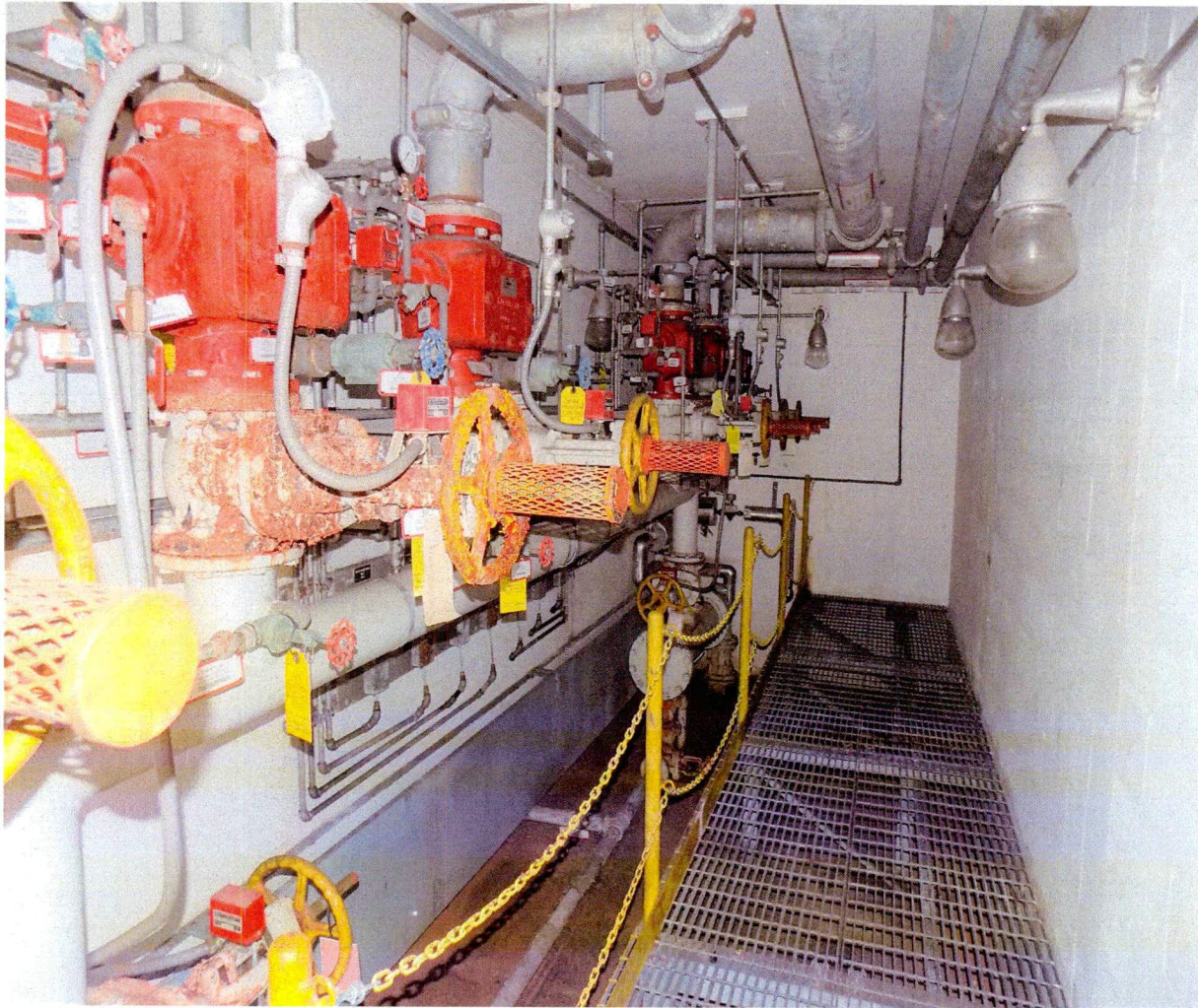
Figure 6. 484-9D Valve Room (Looking East)
