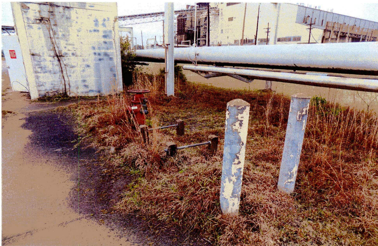
Figure 8. Building 484-9D Hydrant, Support Frame and Bollards
