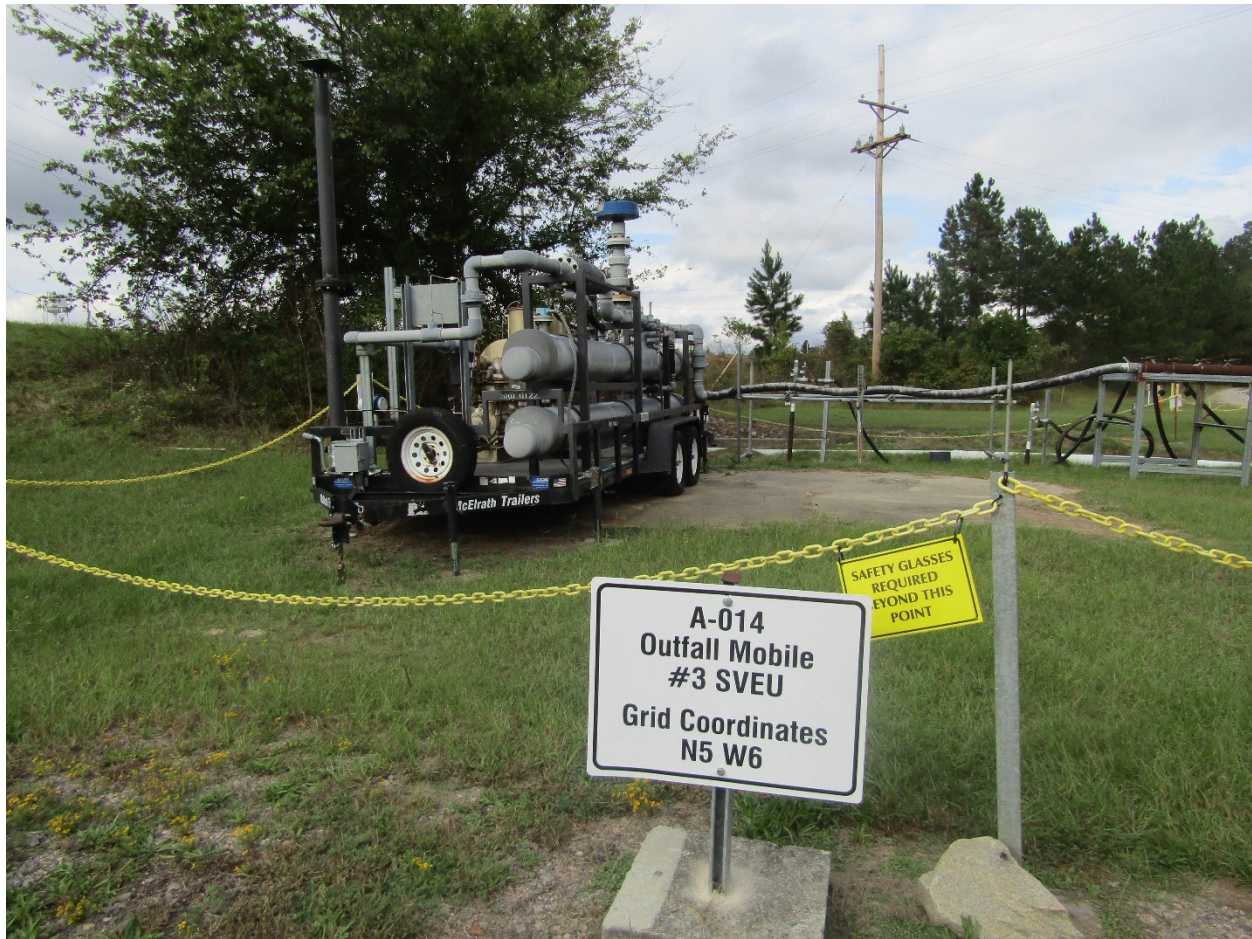
Figure D-5. High Vacuum SVE Unit (i.e., Mobile #3) at A-014 Outfall (2017)
