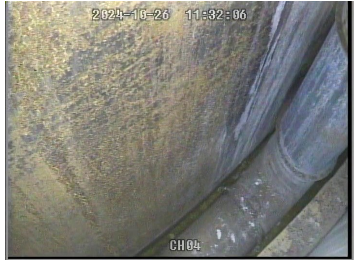
Dehumidification Duct West Side
