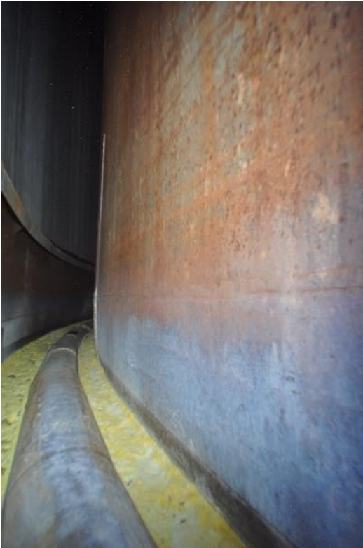
East Riser Facing South
