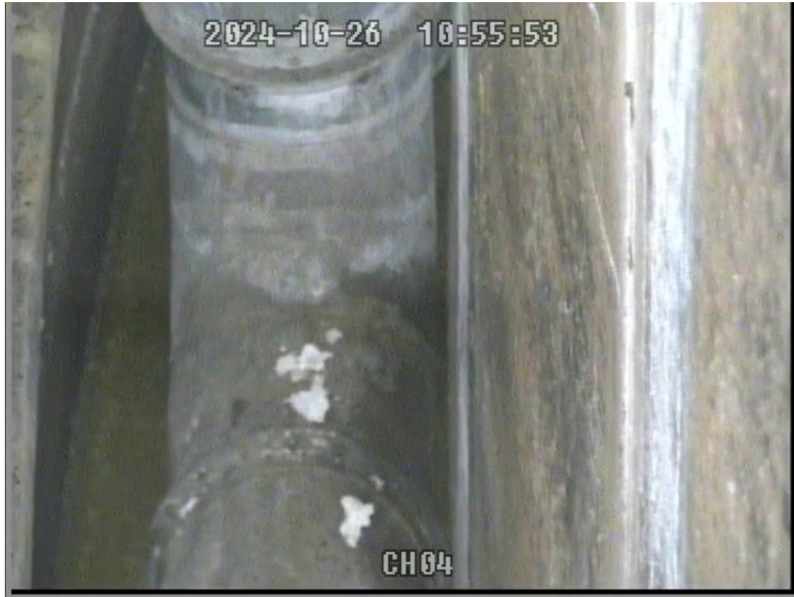
Dehumidification Duct South Side
