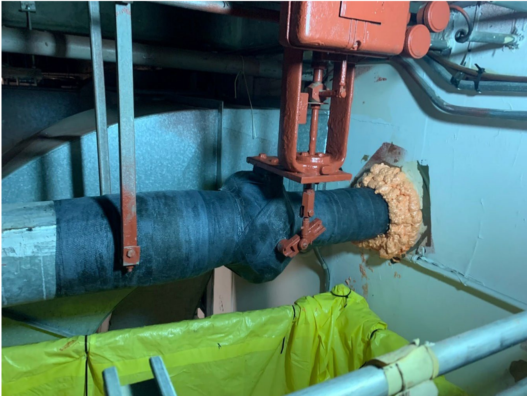
Figure B10 – Sealed Ductwork, ABL Exhaust, Room 2007, East Wall
