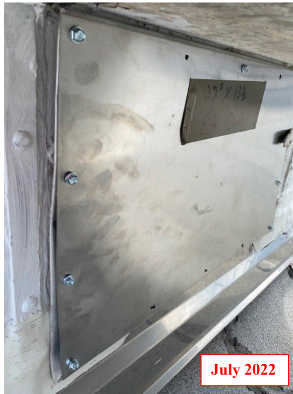
Figure B12 – Covered Outlet for E4 Exhaust Fan (Roof of Building 235-F)
