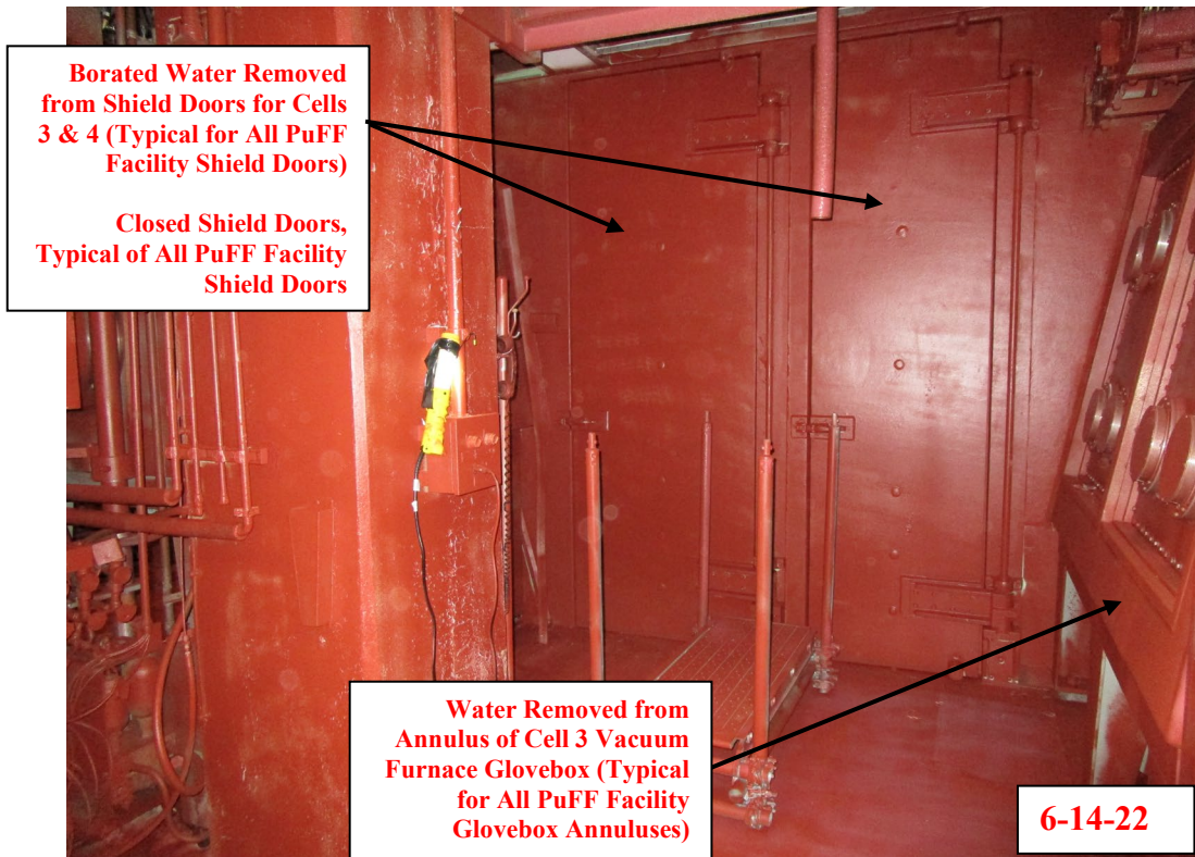
Figure B13 – Drained Shielding and Shut Shield Doors in Room 1002
