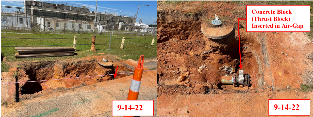
Figure B7 – Air-Gapped Domestic Water Line to 235-F, Adjacent to Road South of 235-F
