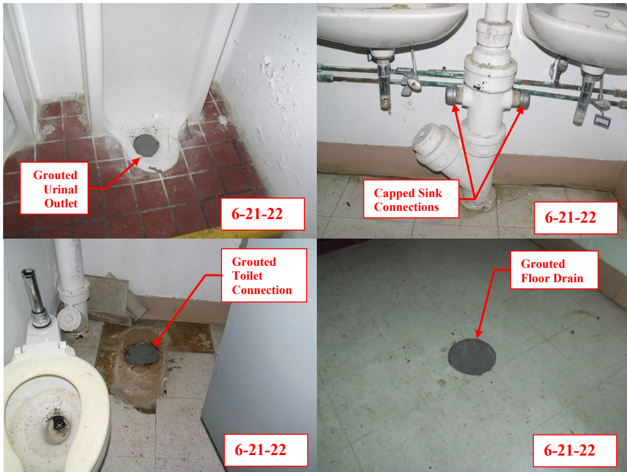
Figure B9 – Sealed Sanitary Sewer Connections in 235-F (Typical)
