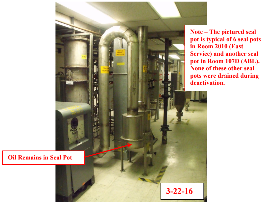
Figure B21 – Undrained Seal Pot in Room 2009 for PuFF Facility Cell 9
