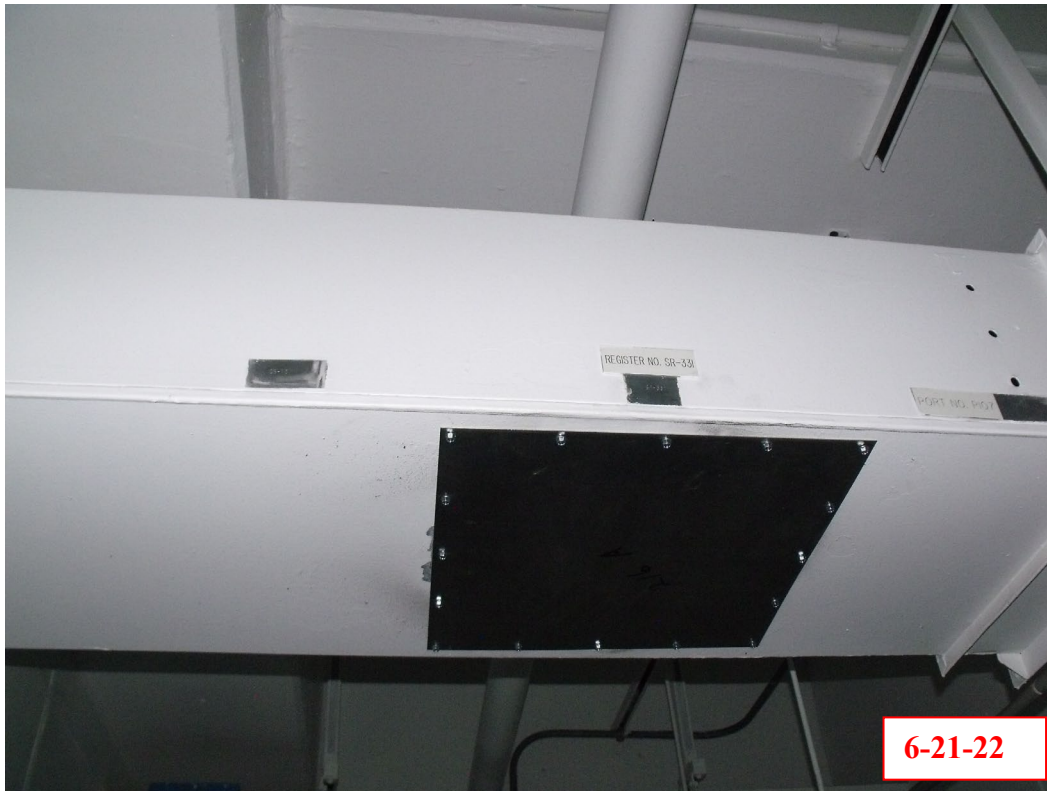
Figure B11 – Sealed Register to the E5 Exhaust System, Room 216A
