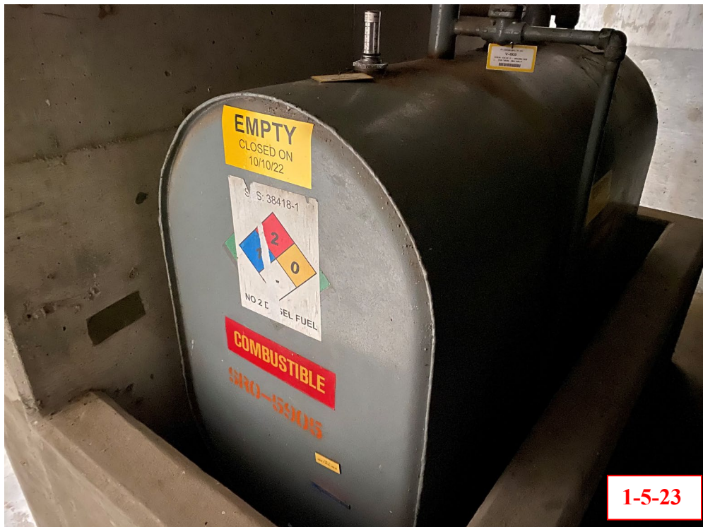
Figure B17 – Drained and Isolated Storage Tank for Diesel Fuel, Southeast Corner 235-F
