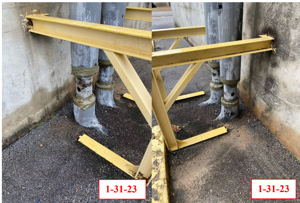
Figure B8 – Air-Gapped (Hole Installed) Chilled Water Lines on West Exterior Wall of 235-F
