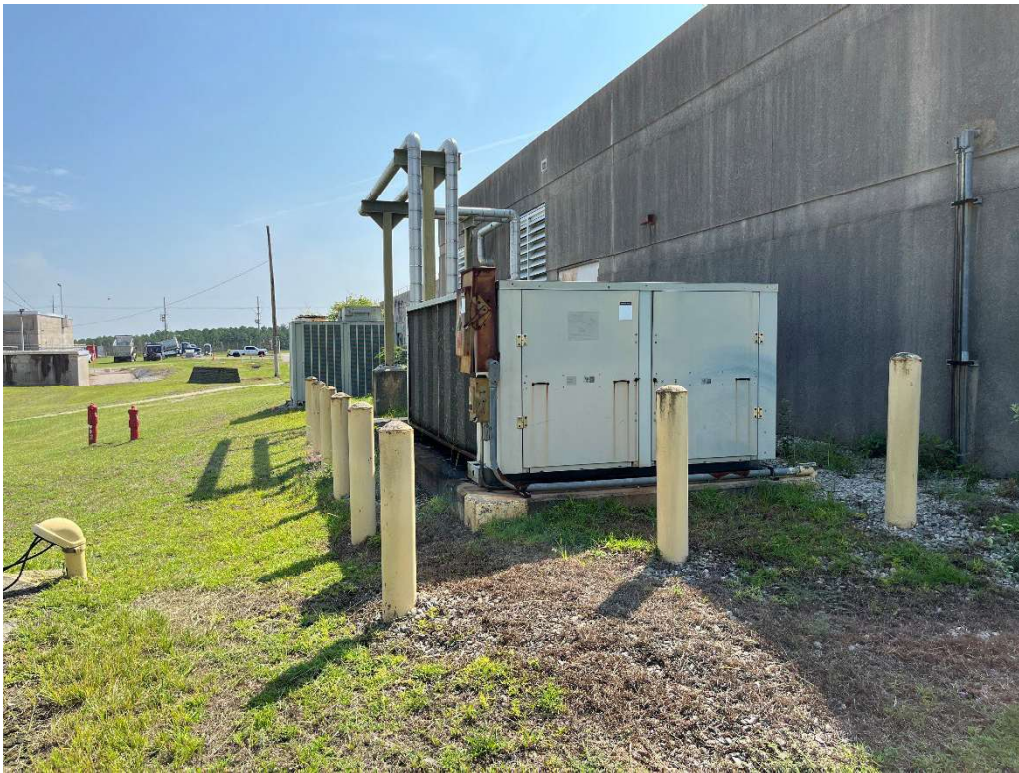
Figure 5: North Side of CAS Featuring the A/C Units and Slabs.
