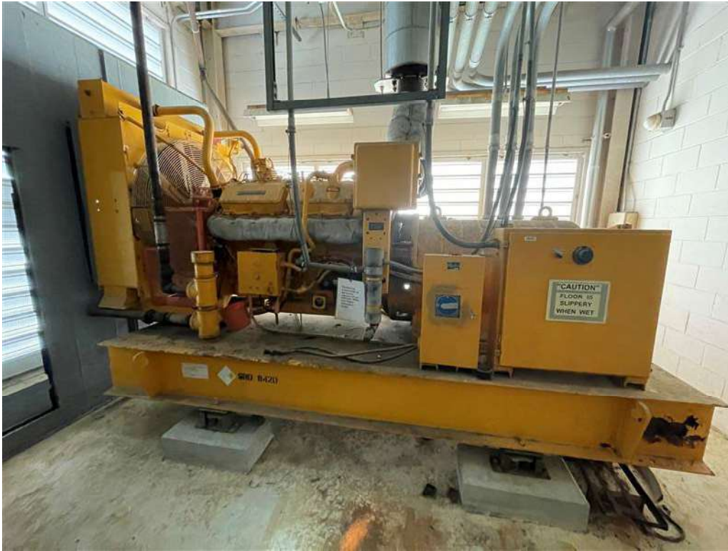
Figure 4: Diesel Generator within 720-F.
