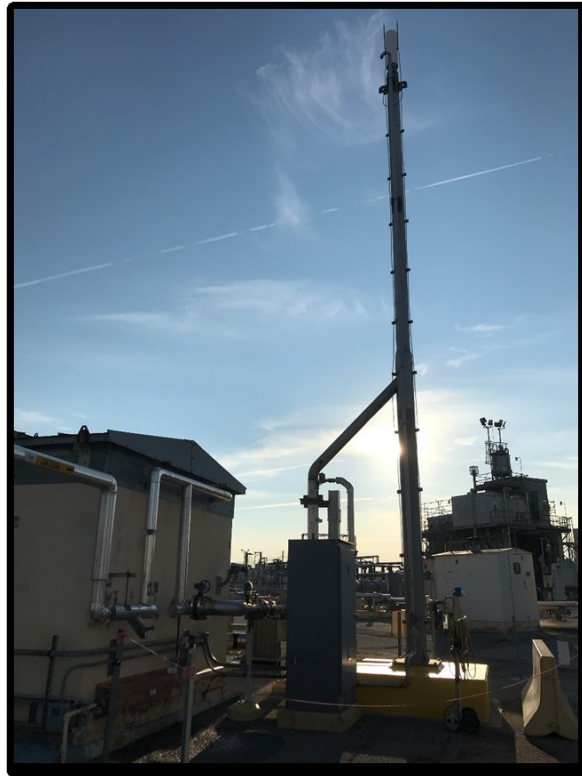
Figure 14: Tank 44F H&V Stack Extension
