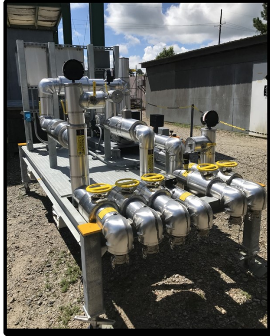
Figure 9: Tank 27F Water Addition Skid
