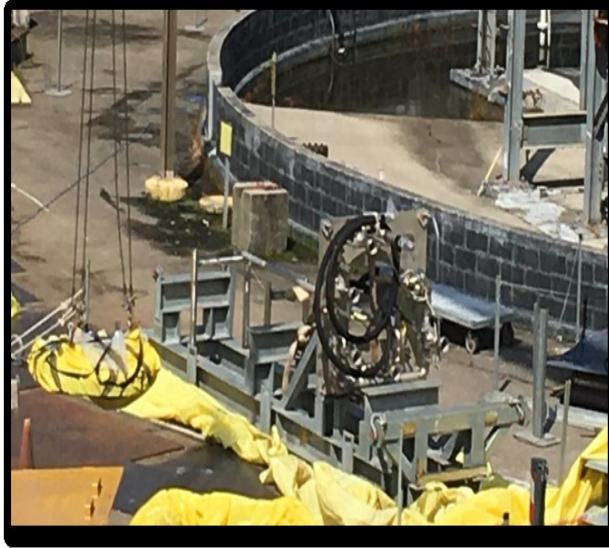
Figure 5: Tank 9H STP Manifold
