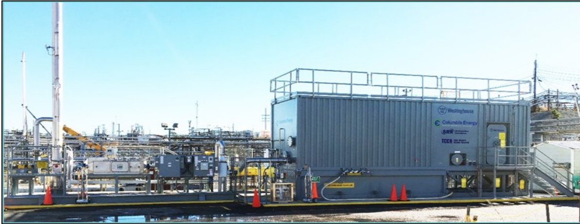
Figure 1: TCCR Process Enclosure and Ventilation Equipment
