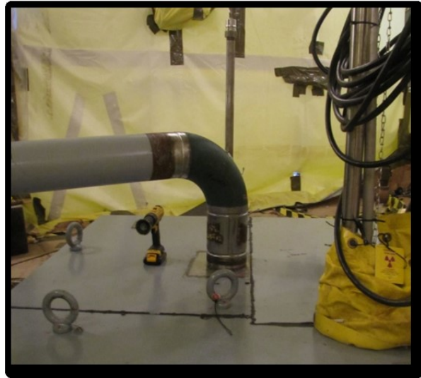
Figure 8: Tank 27F Transfer Line
