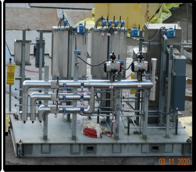
Figure 6: Tank 9H GRM Skid
