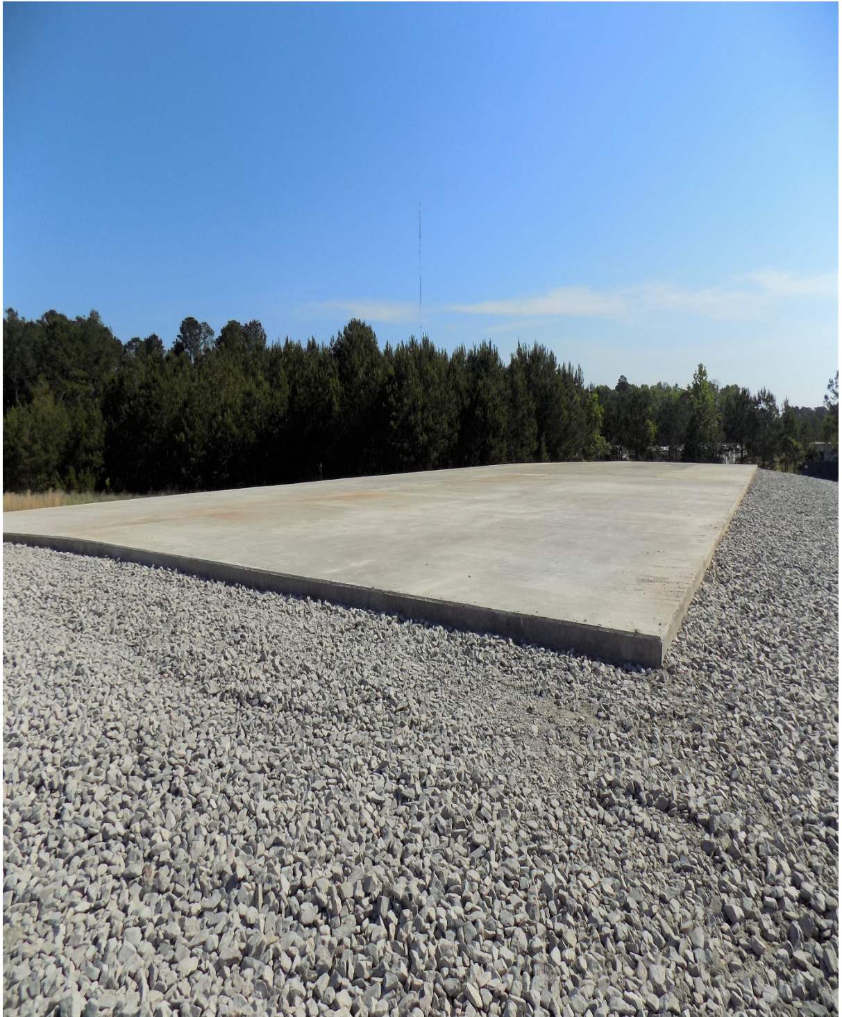
Photo 2 – Building 690-N, Process Heat Exchanger Repair Facility (Looking Northeast) After Decommissioning and Installation of Cap Slab
