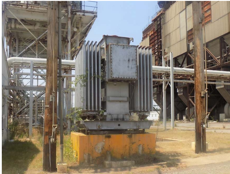
Figure 5. Transformer AT2W (Drained & Disconnected)
