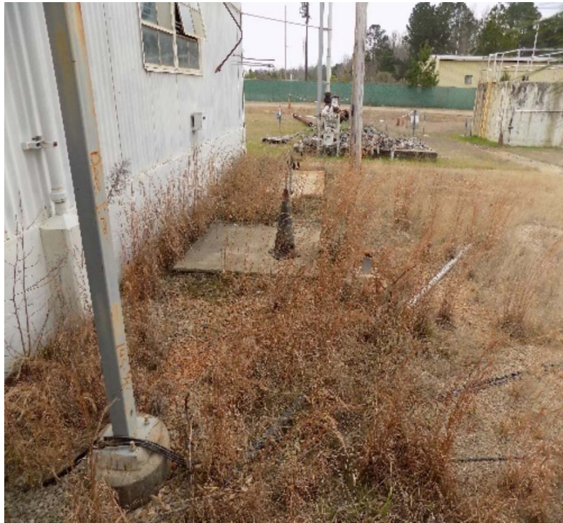
Figure 8. Old Location of Transformer W4
