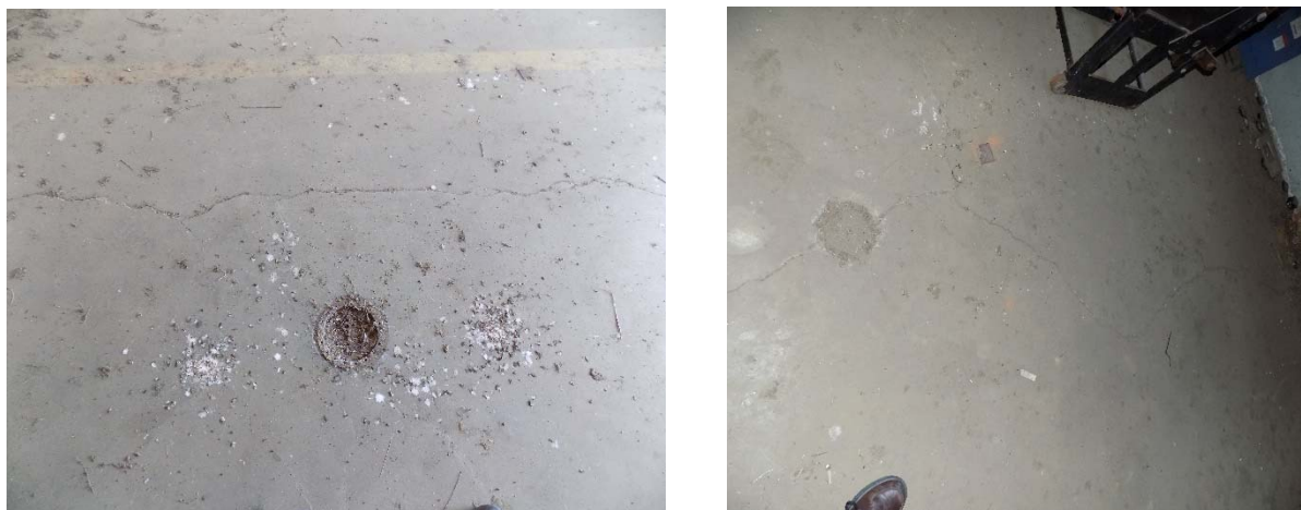
Figure 4. Floor Cracks In Proximity To Clean out And Drains
