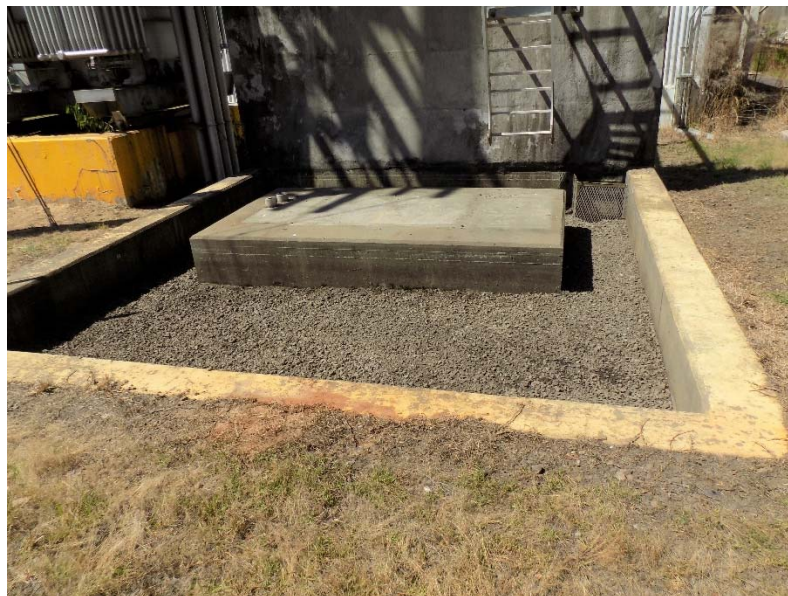
Figure 6. Transformer AT1W Transformer Pad Location with Containment Dike
