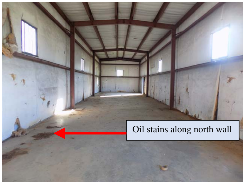
Figure 4. Building 484-15D, D-Area Storage Building Slab Stains
