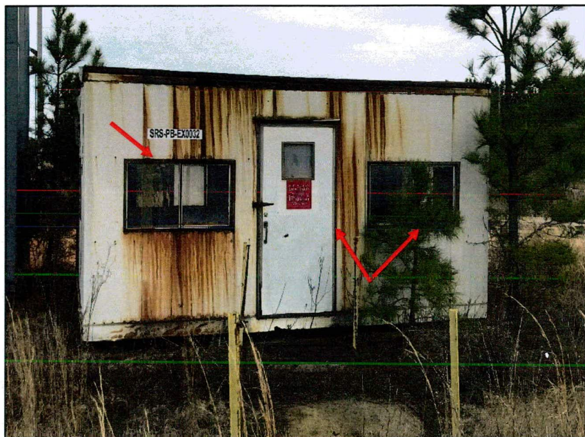
Photograph 1. View facing northeast. Red arrows point to sealant (H02OB).
