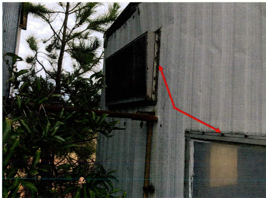
Photograph 3. View facing southeast. Red arrows point to sealant (H02OB).
