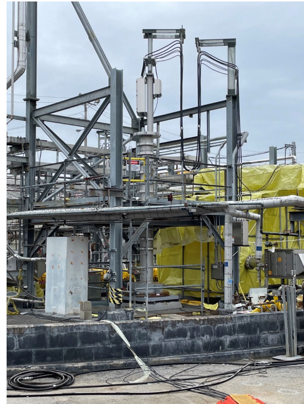
Tank 10 Riser 4 CSMP
