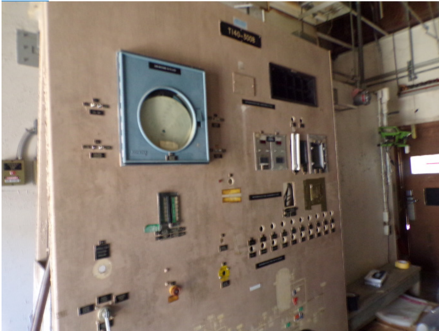
Figure 5. Control Room Panel Post Deactivation
