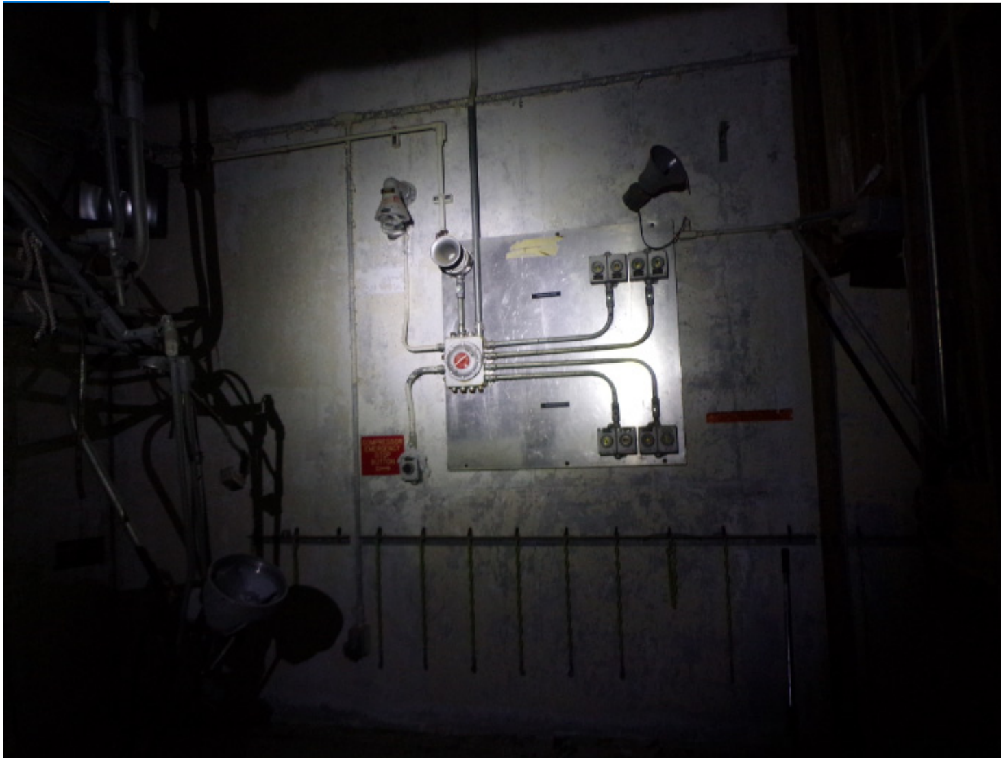
Figure 7. Alarm Panel Post Deactivation
