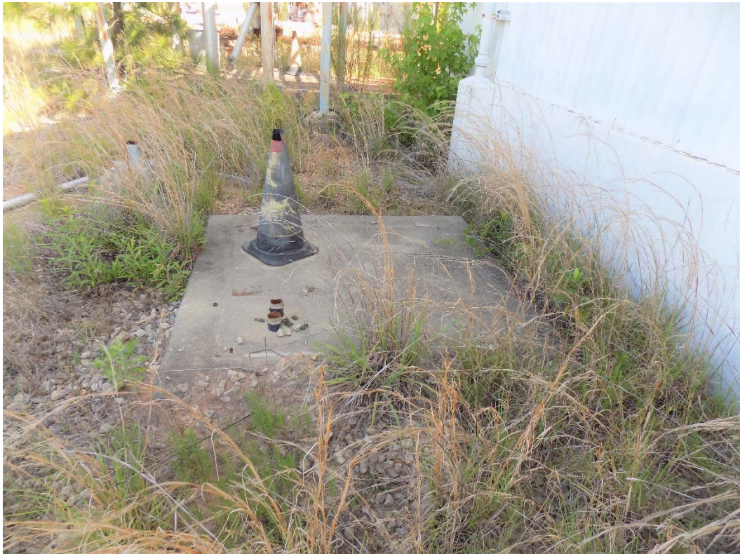
Photo 4: Transformer W4A Concrete Pad Looking North
