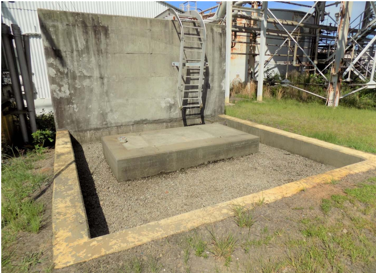
Figure 4B: Transformer AT1W Foundation and Gravel Containment Dike Area Looking Northwest
