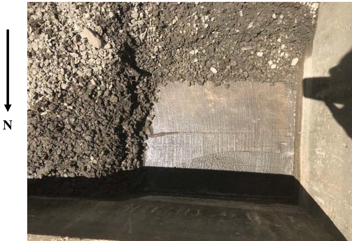
Figure 4C: Transformer AT1W Gravel Containment Dike Area Sump (With Expanded Metal Gravel Barrier Cage Removed) Looking Down Facing South
