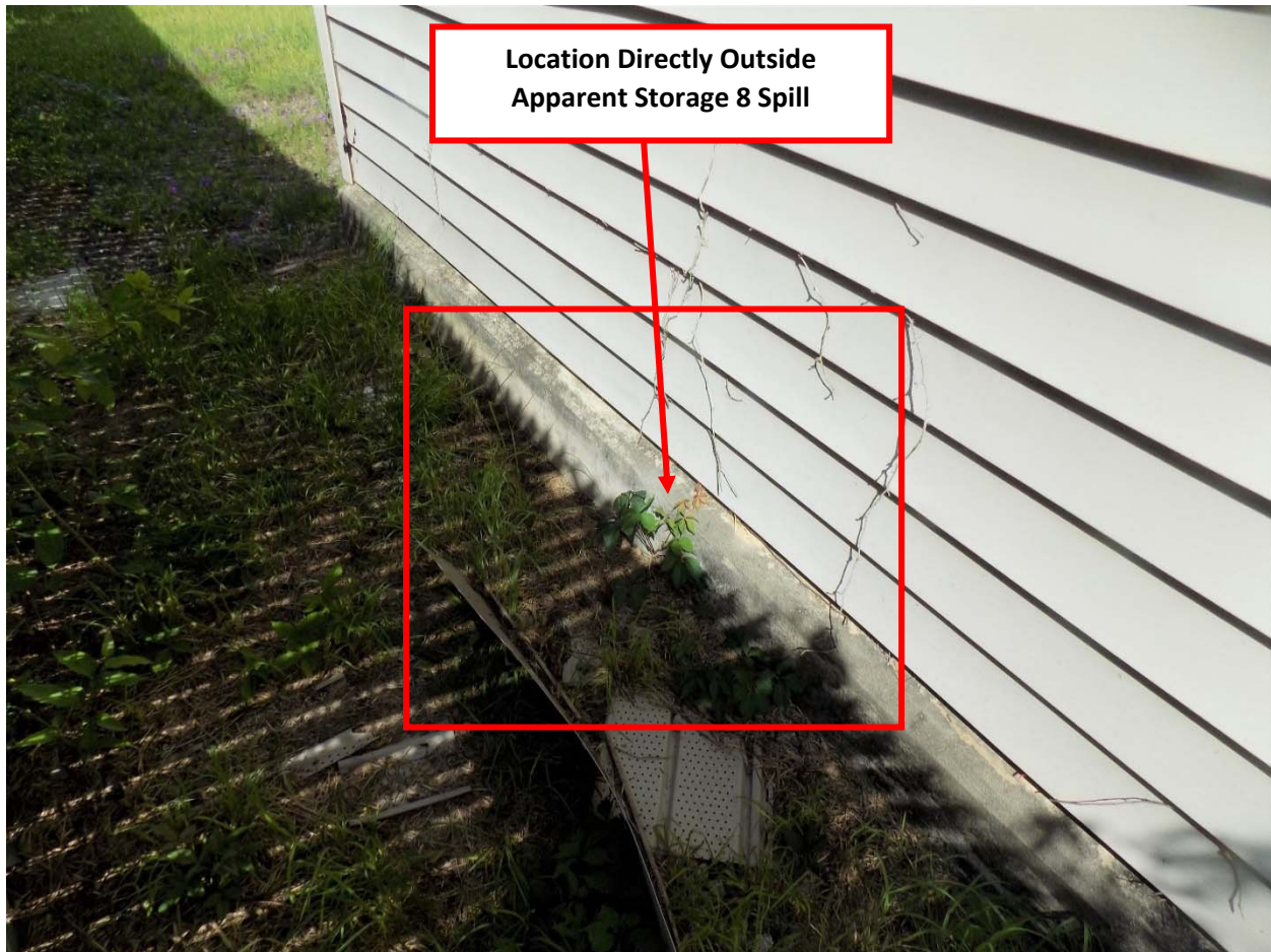
Figure 6C: 710-16D Opposite Side Of Wall From Storage 8 Spill Looking Northwest
