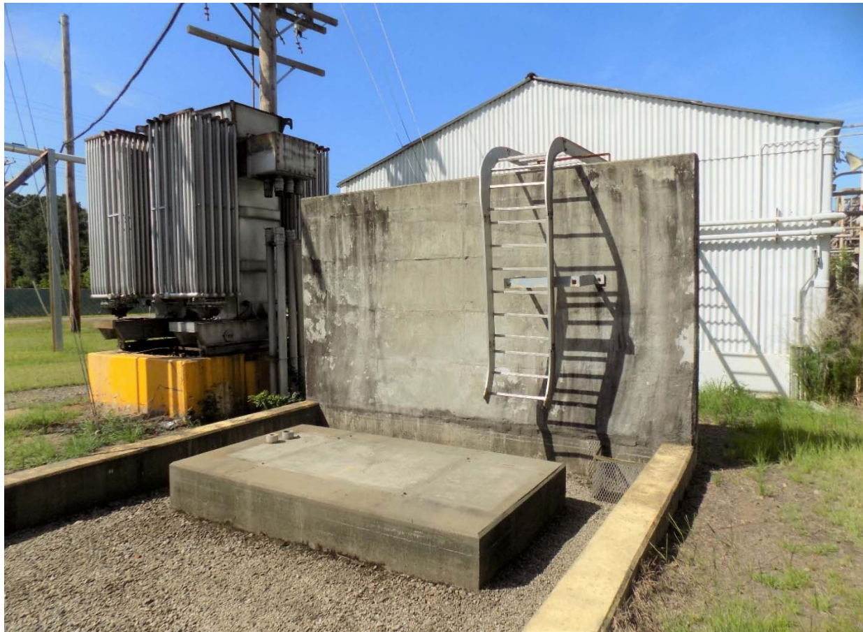
Figure 4A: Transformer AT1W Foundation and Gravel Containment Dike Area Looking Southwest
