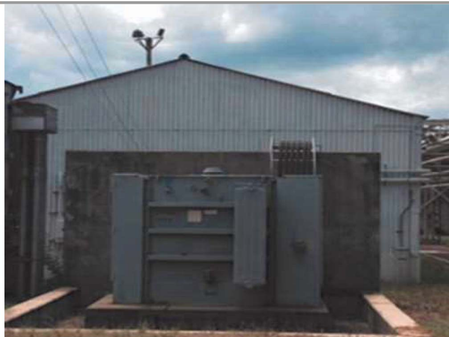
Former Transformer AT1W
