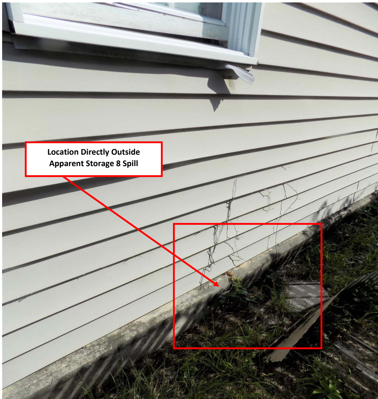
Photo 2 - 710-16D Opposite Side Of Wall From Storage 8 Spill Looking Northeast
