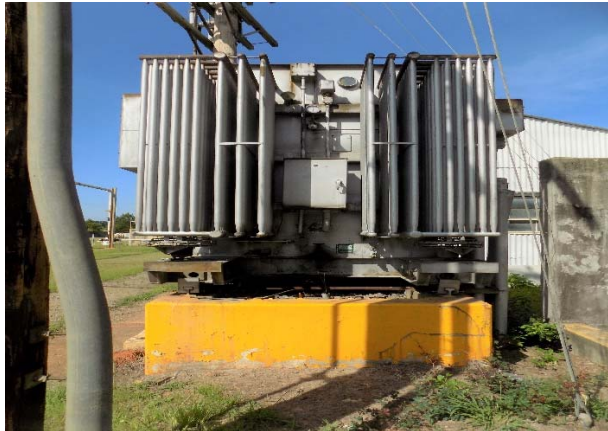
Figure 5B: Transformer AT2W and Pad
