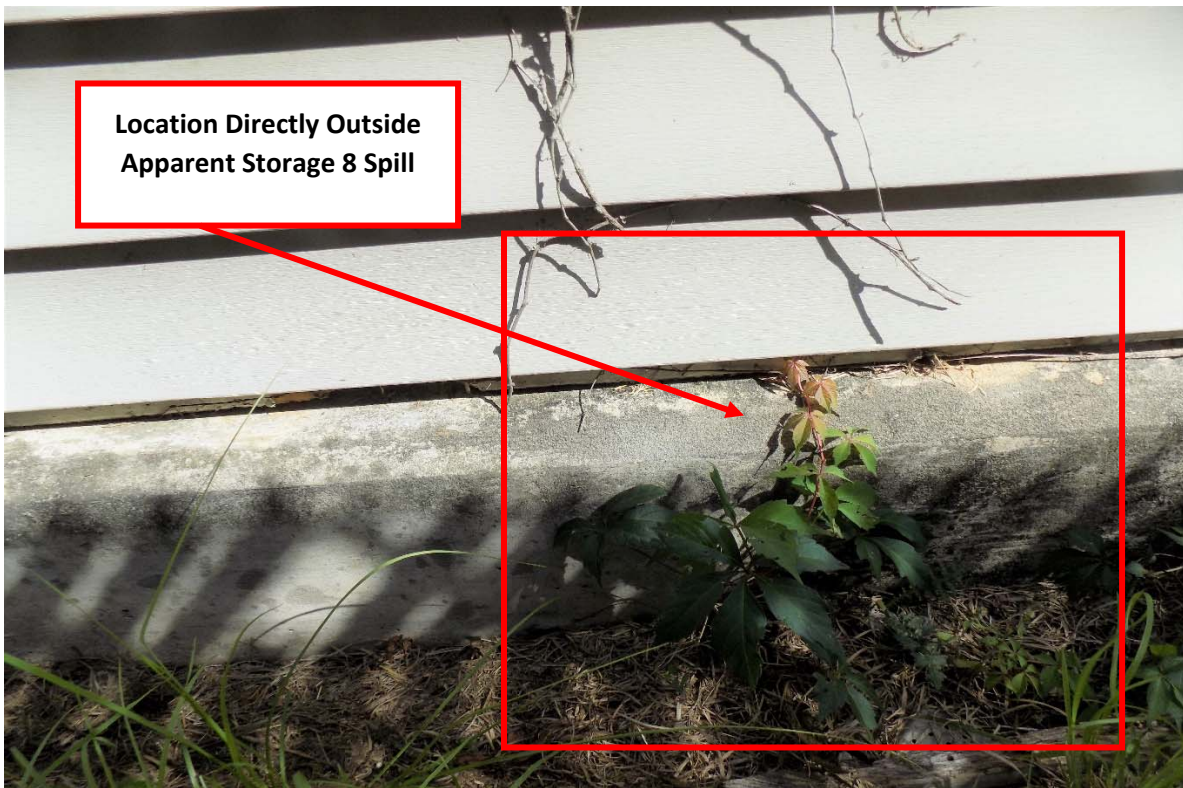
Figure 6A: 710-16D Opposite Side Of Wall From Storage 8 Spill Looking North
