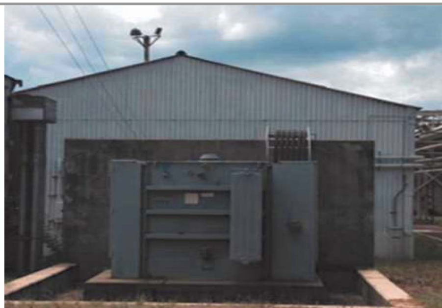
Former Transformer AT1W
