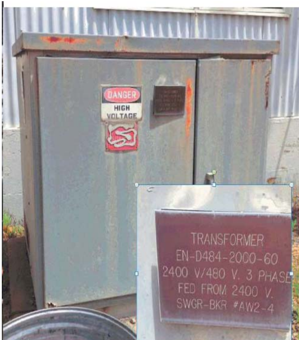
Former Transformer W4A
