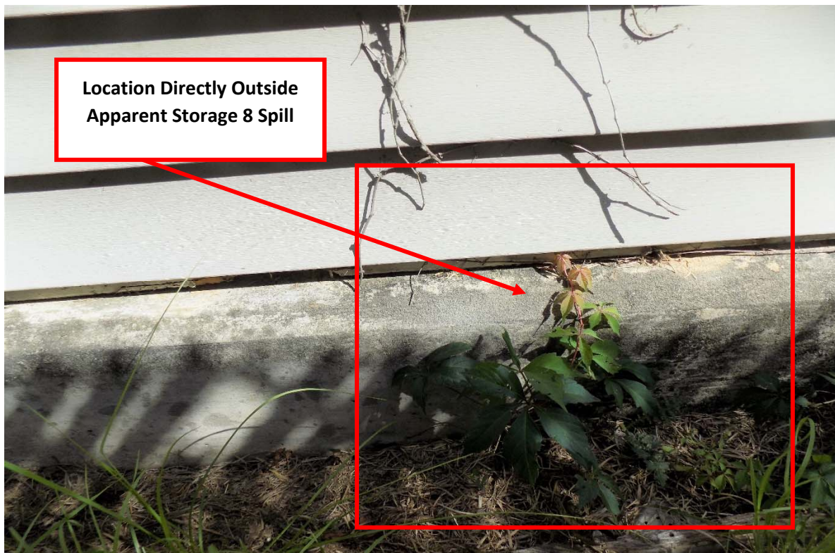
Photo 1 - 710-16D Opposite Side Of Wall From Storage 8 Spill Looking North
