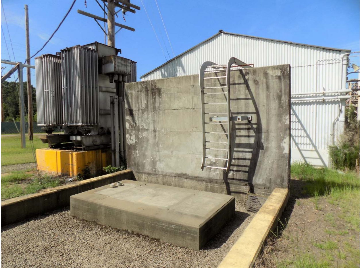
Photo 1: Transformer AT1W Foundation and Gravel Containment Dike Area Looking Southwest
