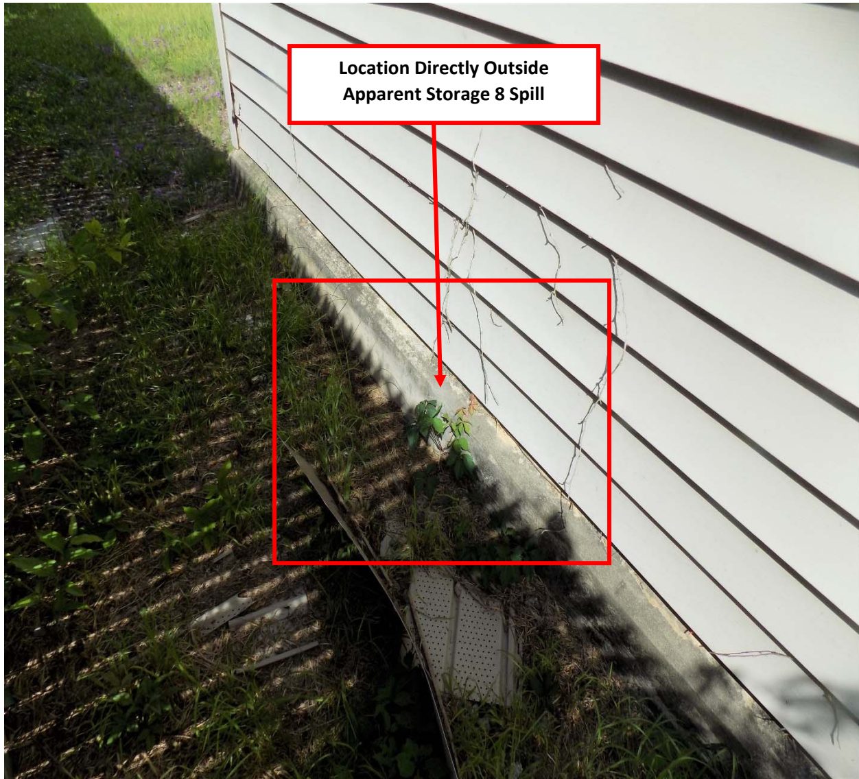
Photo 3 - 710-16D Opposite Side Of Wall From Storage 8 Spill Looking Northwest
