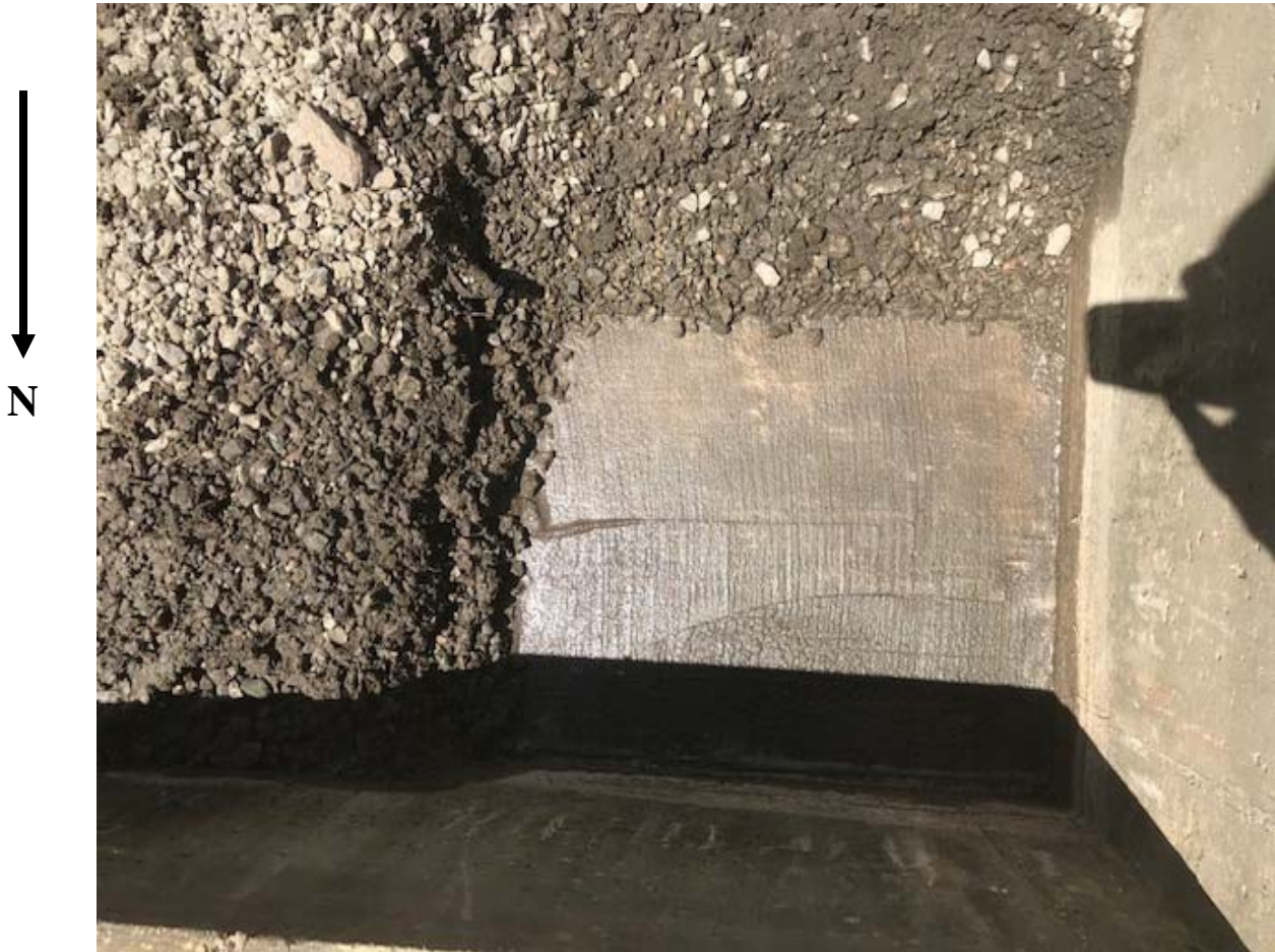
Photo 3: Transformer AT1W Gravel Containment Dike Area Sump (With Expanded Metal Gravel Barrier Cage Removed) Looking Down Facing South
