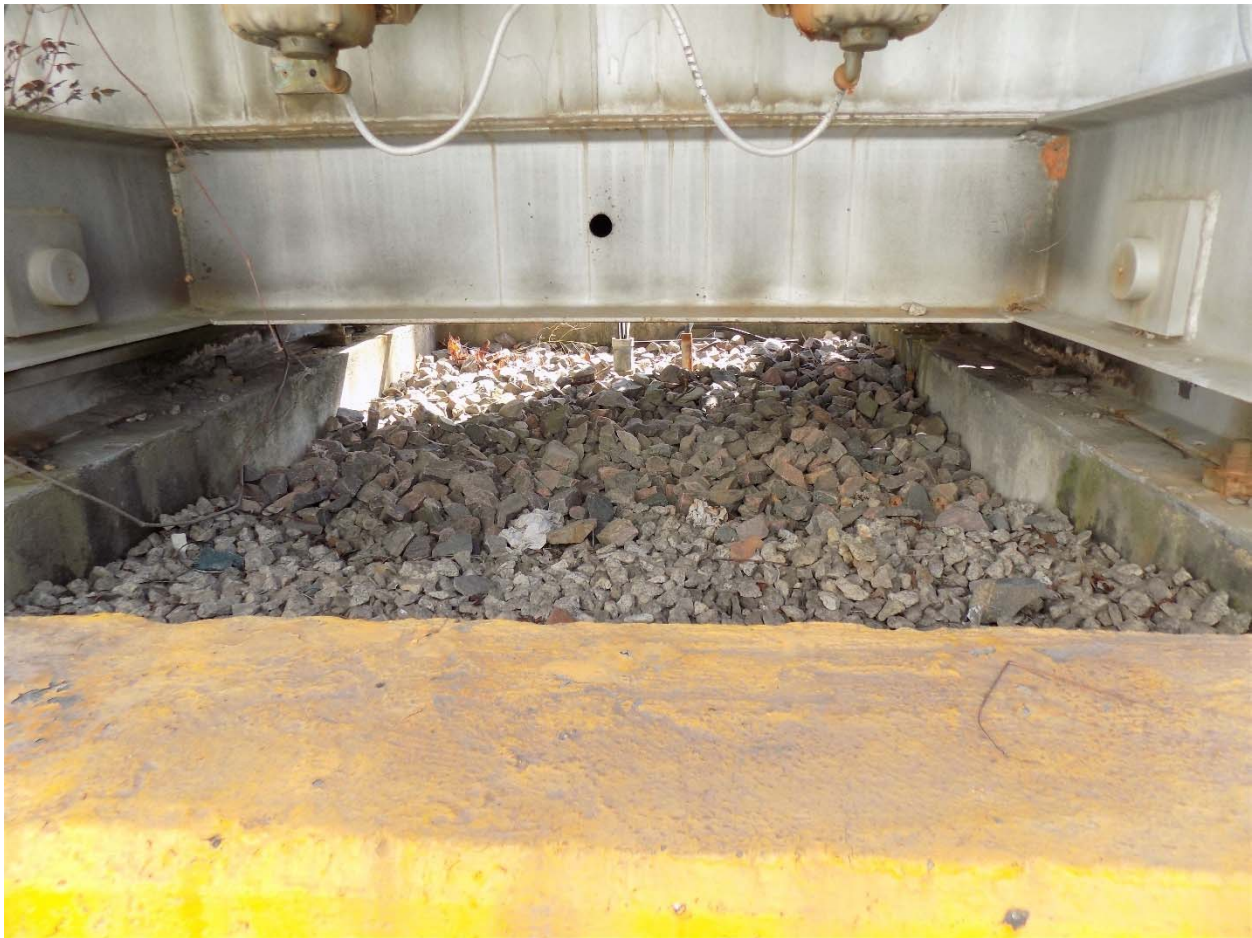
Figure 4E: Pad and Gravel Containment Area Beneath Transformer AT2W
