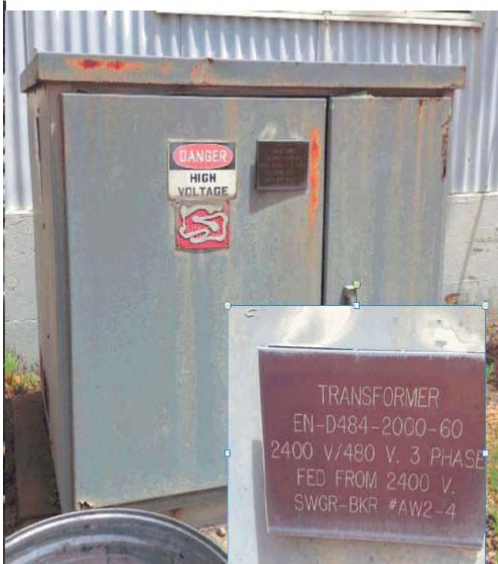
Former Transformer W4A
