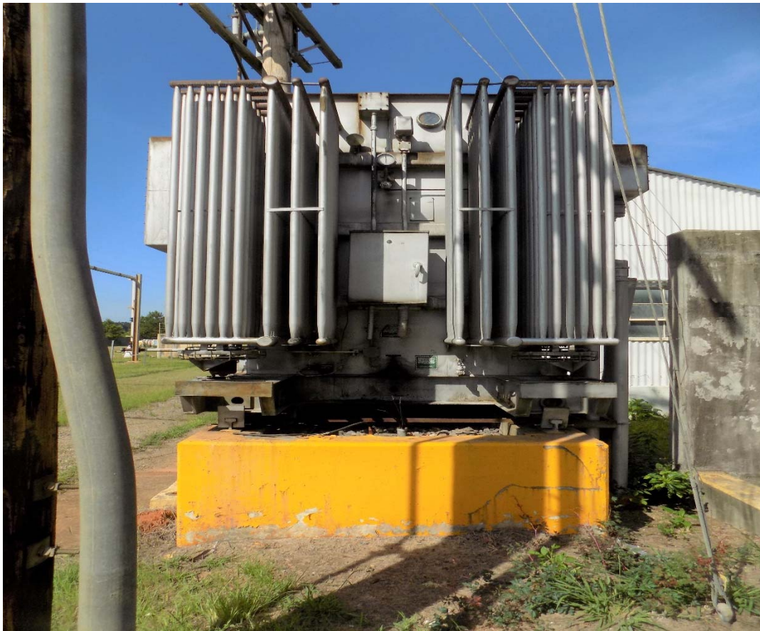
Figure 4D: Transformer AT2W and Pad (Looking West)
