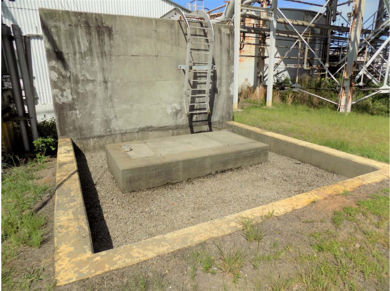
Photo 2: Transformer AT1W Foundation and Gravel Containment Dike Area Looking Northwest
