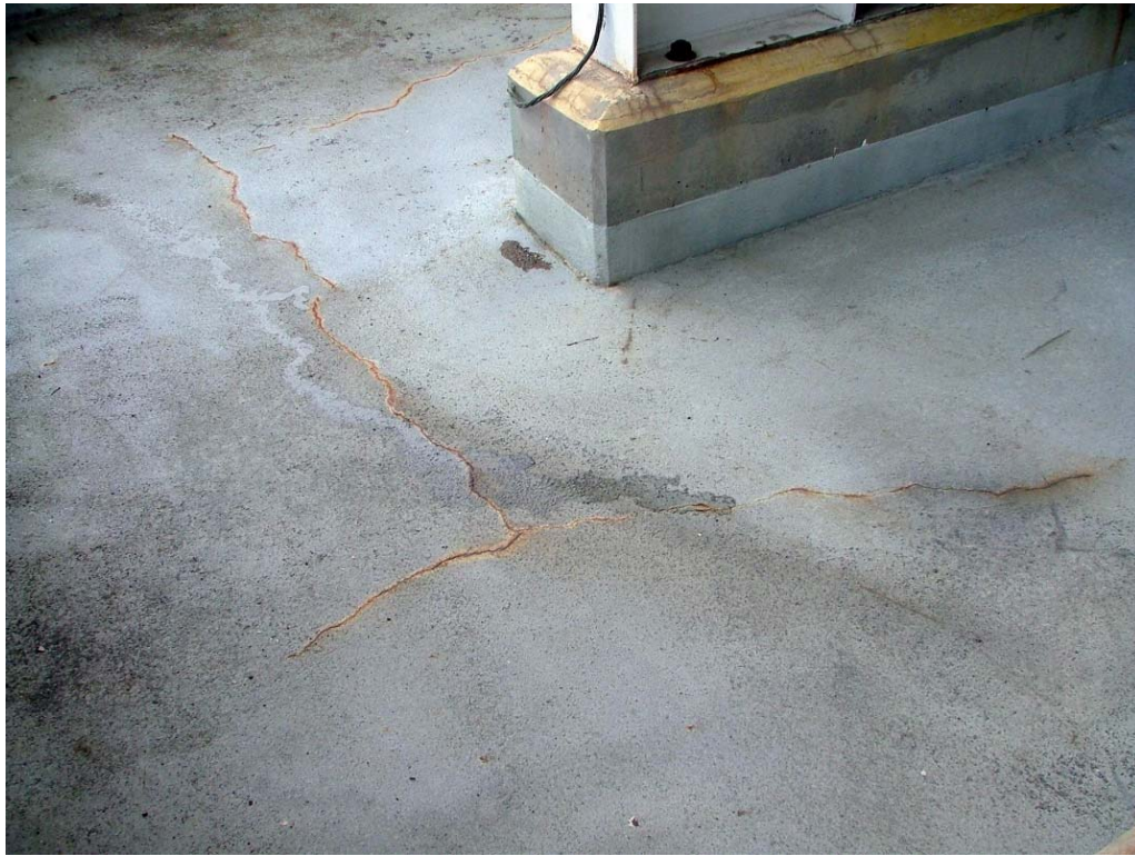
Figure 11. Building 454-D, D-Area Diesel Fuel Tank Minor Surface Slab Cracks
