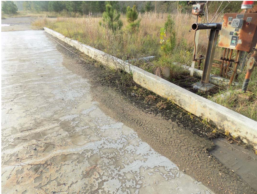
Figure 9. Building 454-1D, D-Area Fuel Unloading Facility (Minor Surface Stains, Cracks and Dirt)
