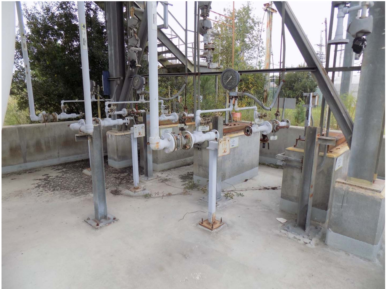
Figure 8. Building 454-D, D-Area Diesel Fuel Tank (Previous Transfer Pump Location)
