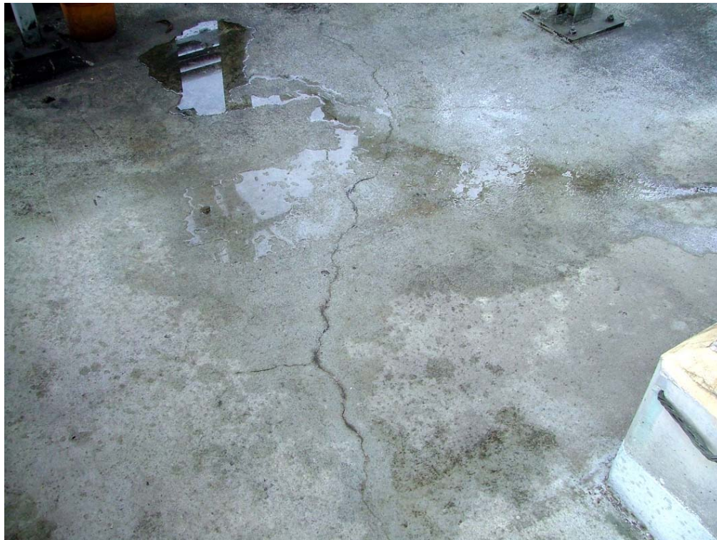
Figure 12. Building 454-D, D-Area Diesel Fuel Tank Minor Surface Slab Cracks and Minor Staining (Northwest End)
