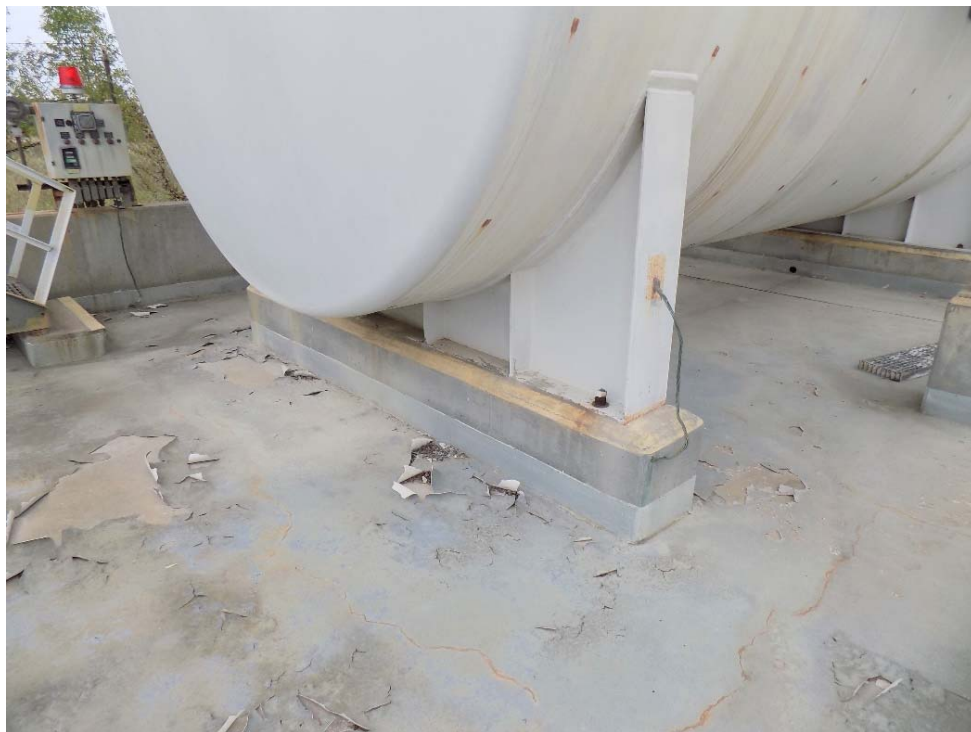
Figure 10. Building 454-D, D-Area Diesel Fuel Tank Minor Slab Cracks and Coating Peeling (South End)
