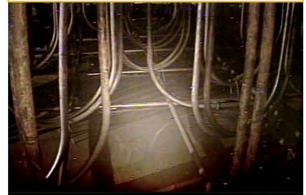
Center Riser to West
