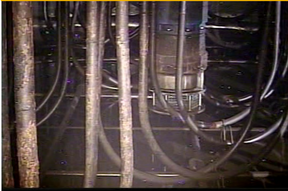
Riser 4 CSMP from Center Riser
