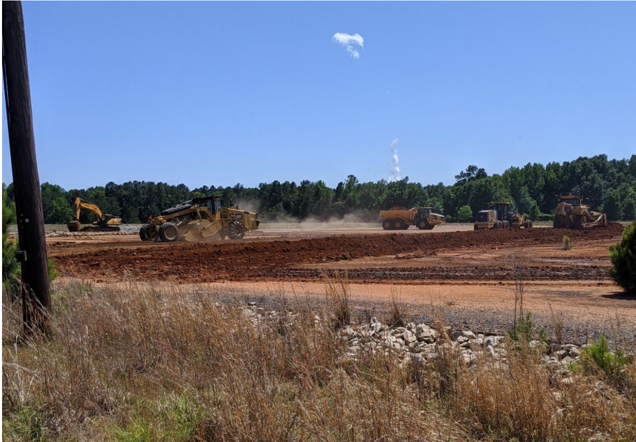
Photo 5. Equipment Types Used (From left to right: excavator, processor, dump truck, grader, and bulldozer work to mix amendment)
