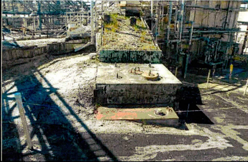
Tank 18, Southwest Riser
