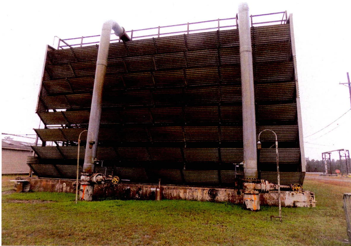
Figure 5. Building 485-D, D-Area Cooling Tower Water Return Lines
