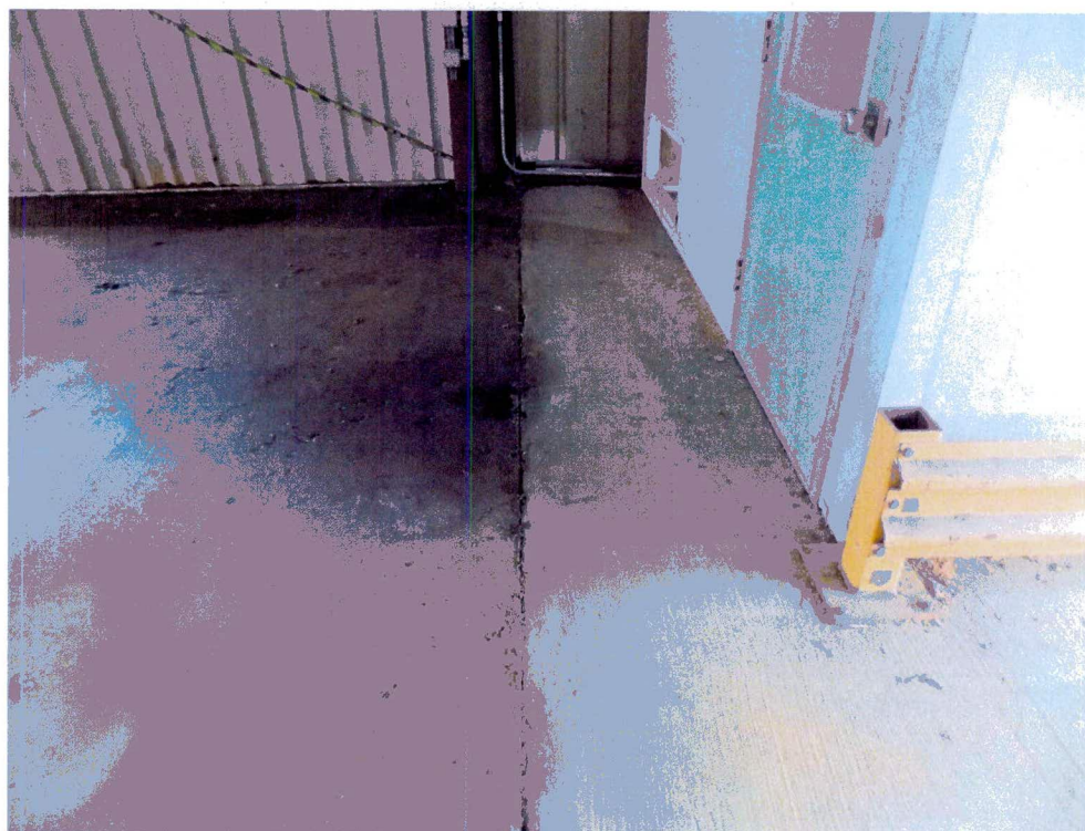
Figure 6. Building 484-13D, D-Area Storage Building Floor Stain
