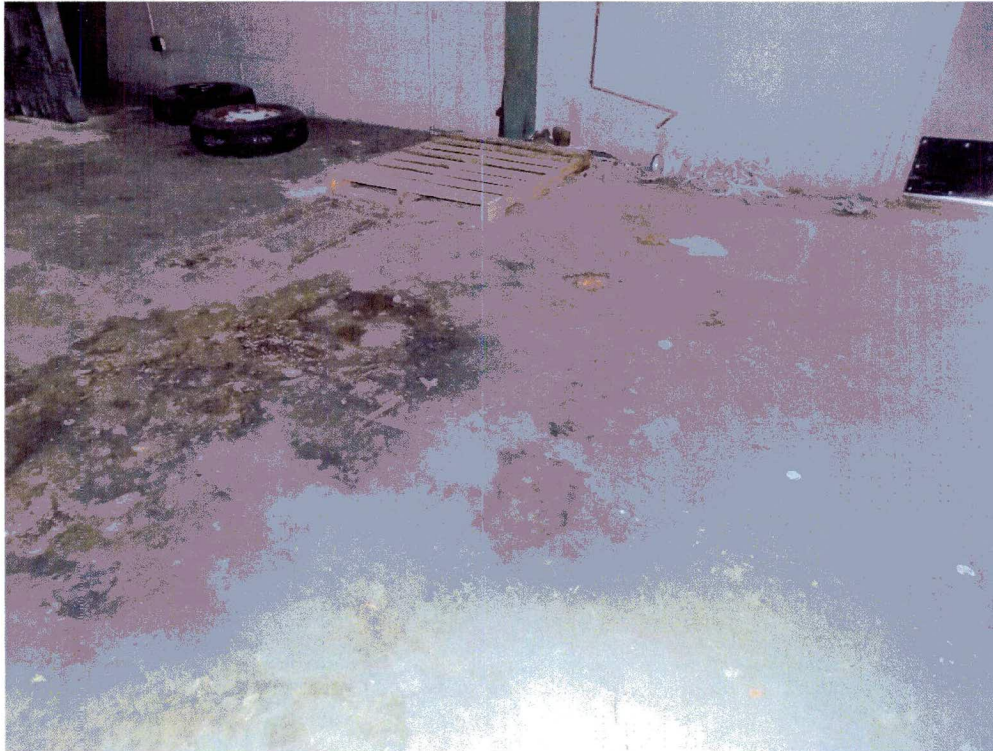
Figure 1. Stained Concrete Near East Door
