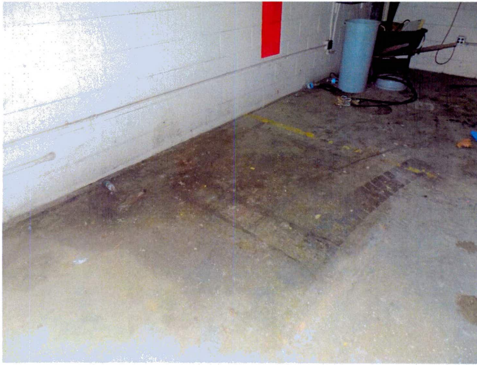
Figure 2. Stained Concrete Near Wall Perpendicular to South Wall
