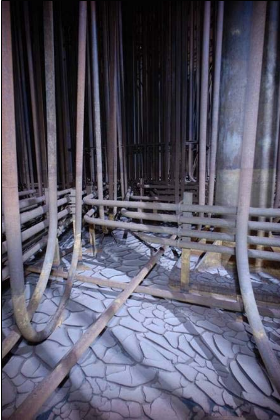
Figure 2.2-4: Type I Tank (Tank 5F) Cooling Coils
