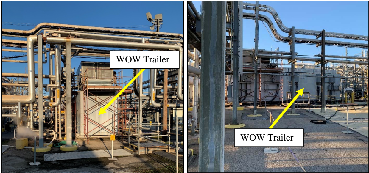
Figure 4.3-5: WOW Control Trailer
