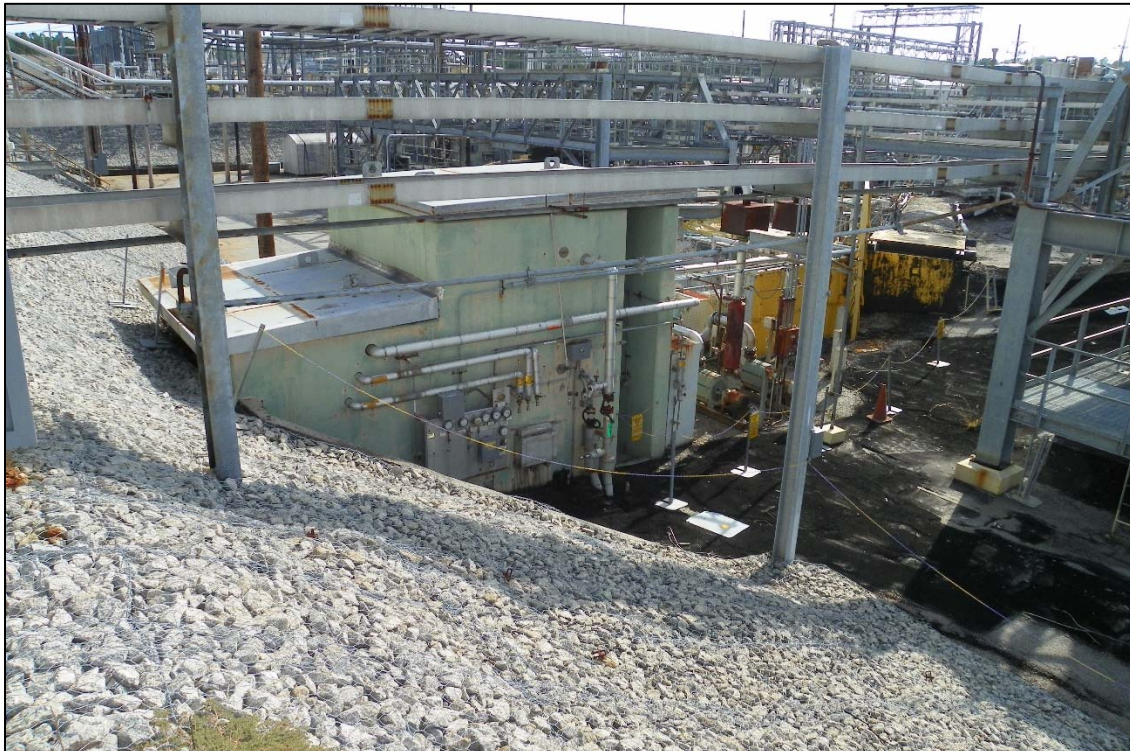
Figure 4.2-12: View from above the Ventilation System
