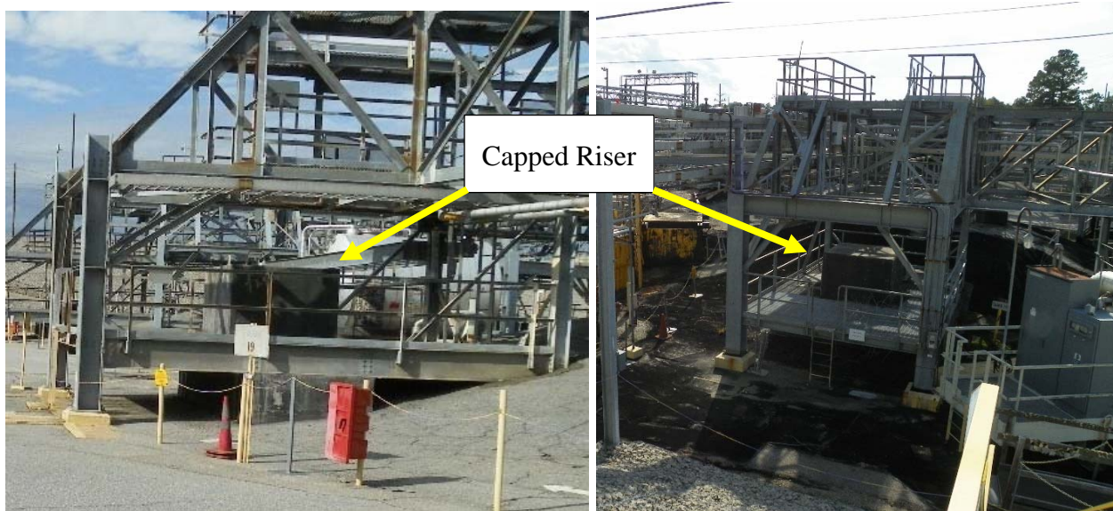
Figure 4.2-2: Examples of Capped Waste Tank Risers
