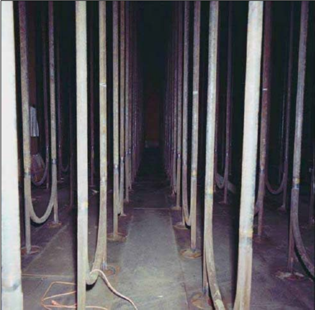
Figure 2.2-11: Cooling Coils in a Type IIIA Tank
