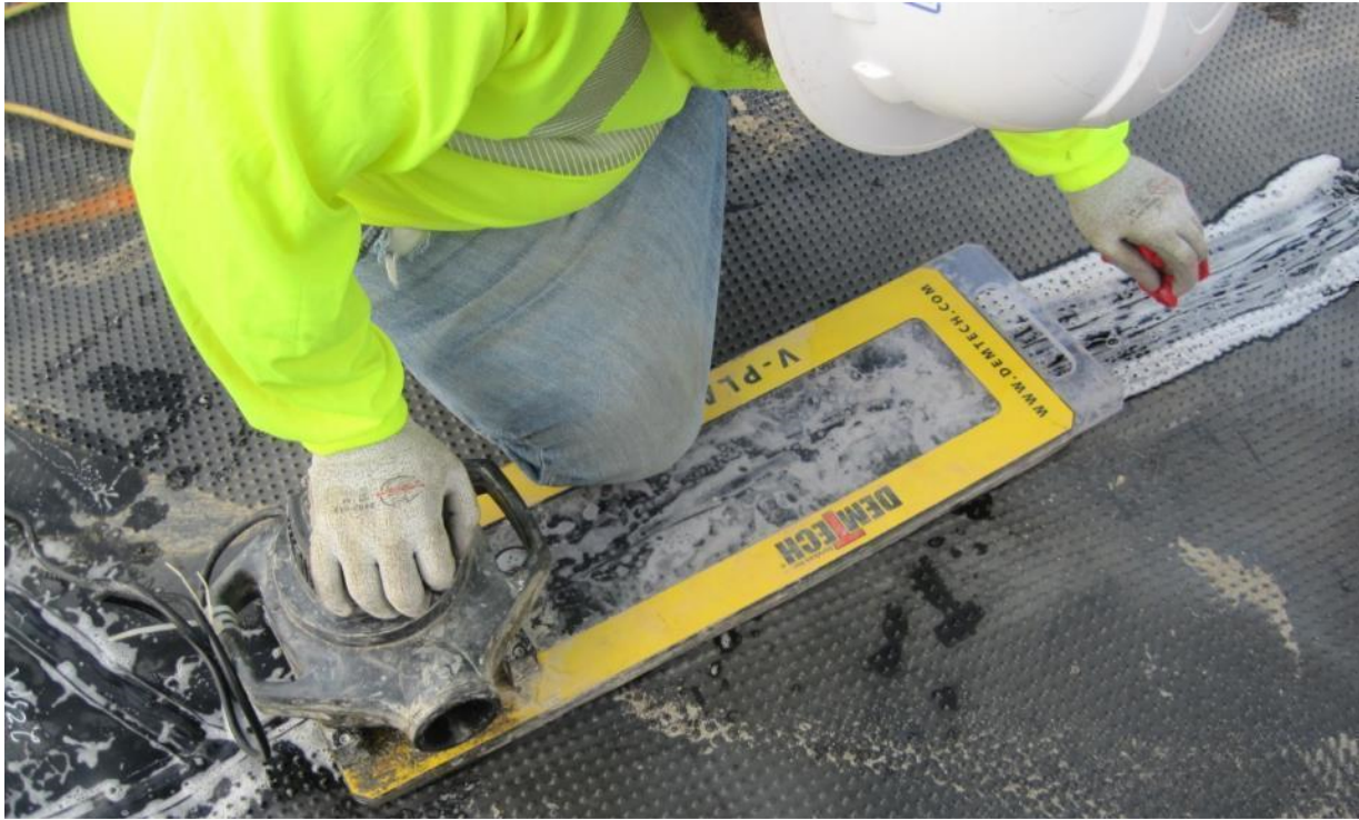
Photo 21. Vacuum Testing of Extrusion Weld
