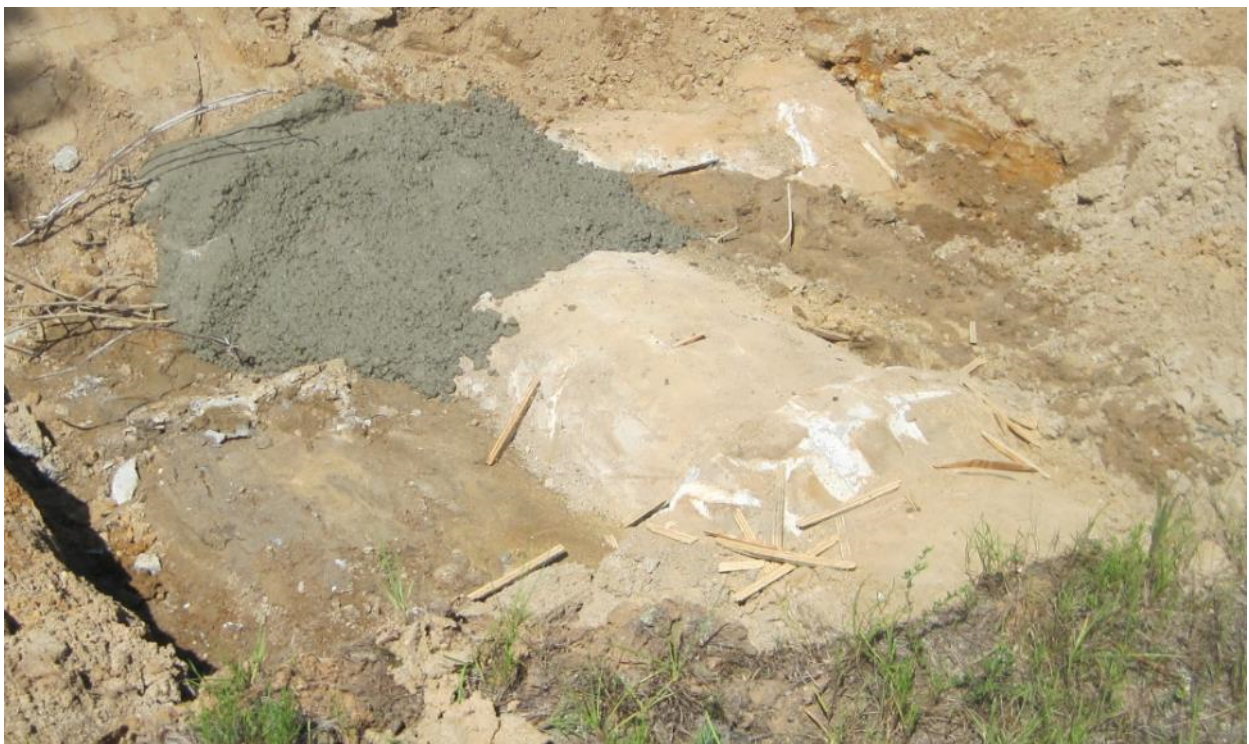
Photo 38. 489-D CPRB Plugged 48" Pipe
