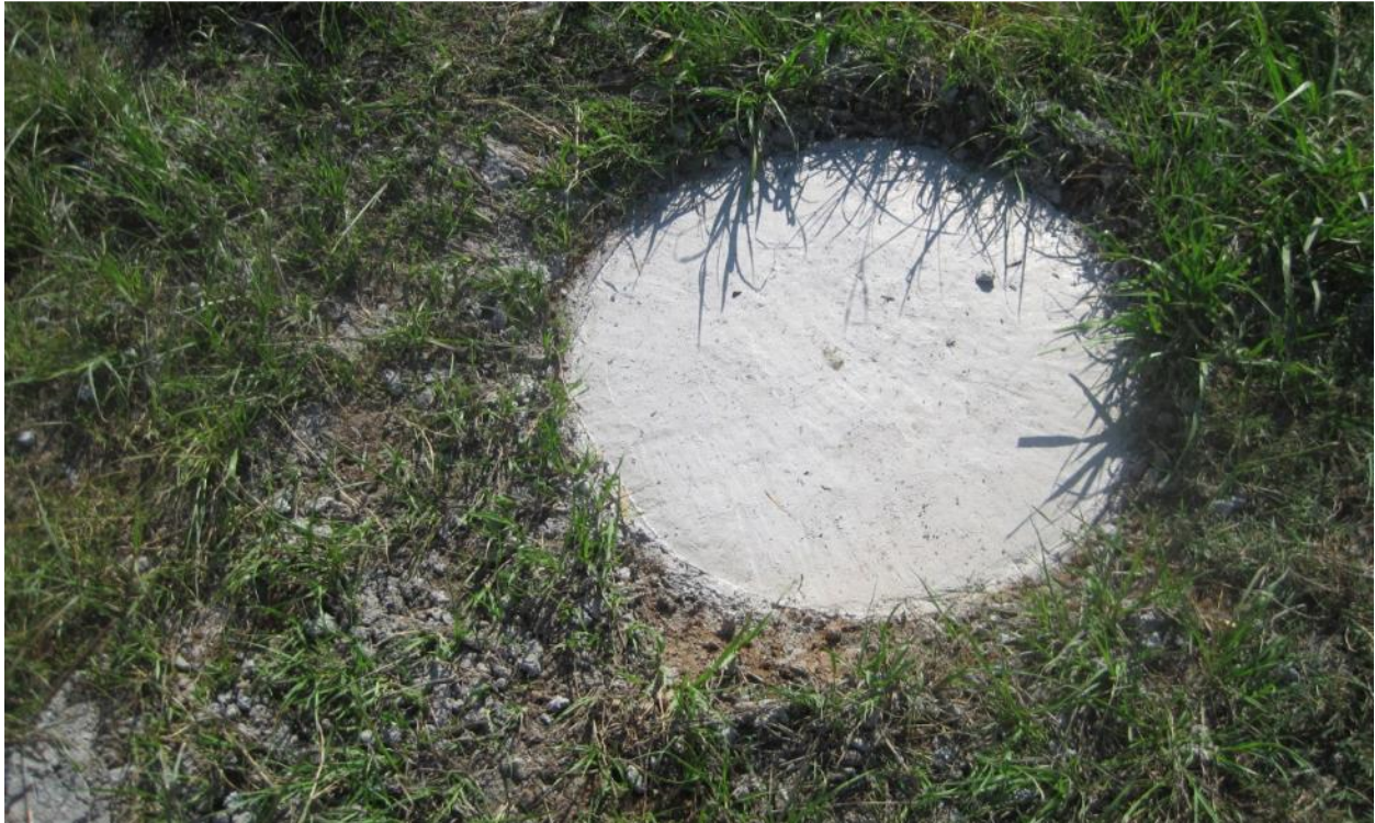
Photo 37. 489-D CPRB Plugged Manhole (Typical for 2)
