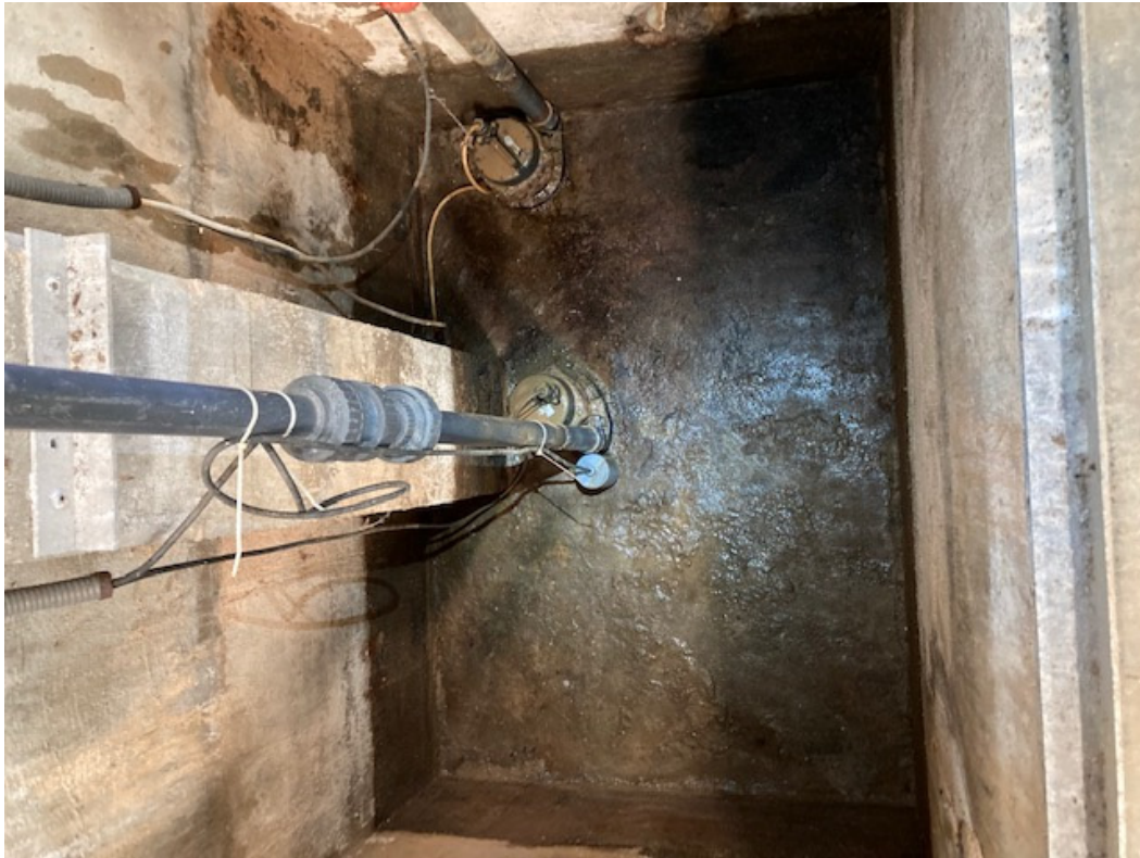
Figure 1: Photo of Bottom of Sump in 483-7D
