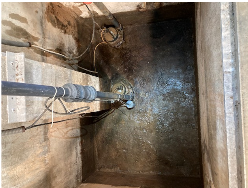
Figure 2. Photo of Bottom of Sump in 483-7D
