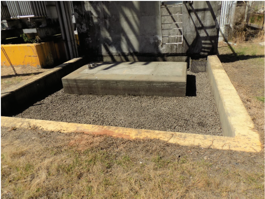
Figure 8. Transformer AT1W Transformer Pad Location with Containment Dike
