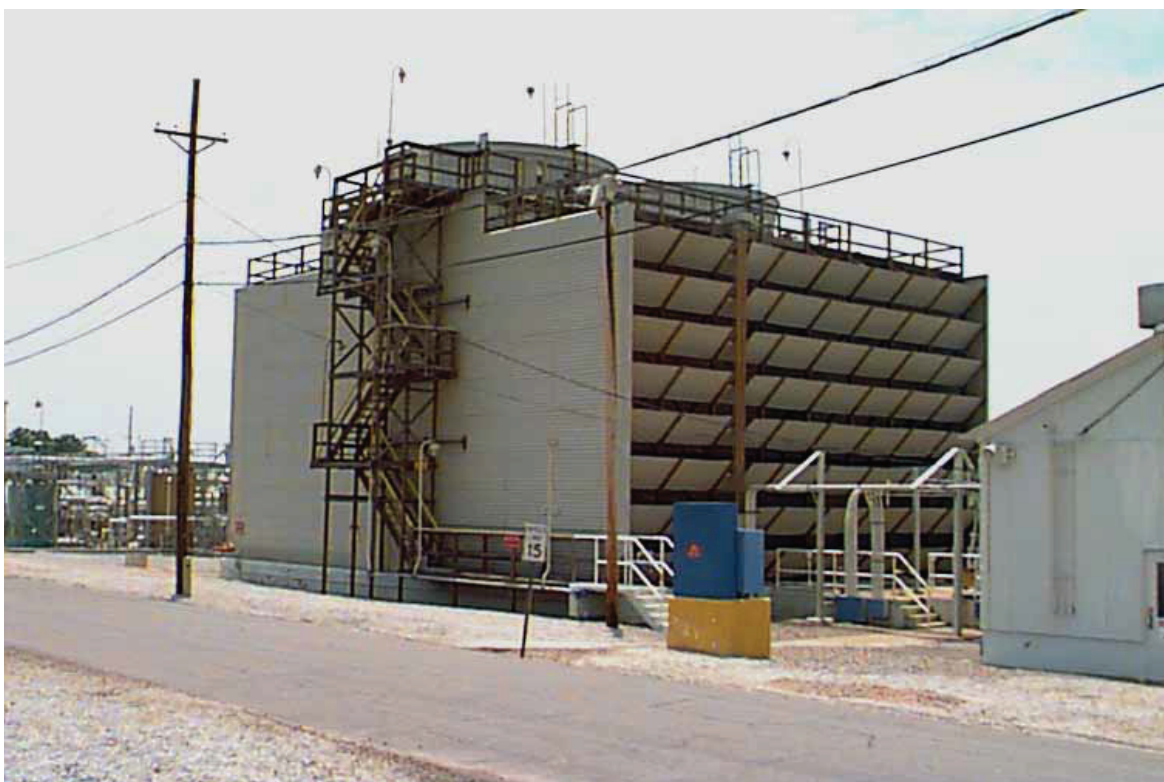
Figure 22. Building 485-D, D-Area Cooling Tower
