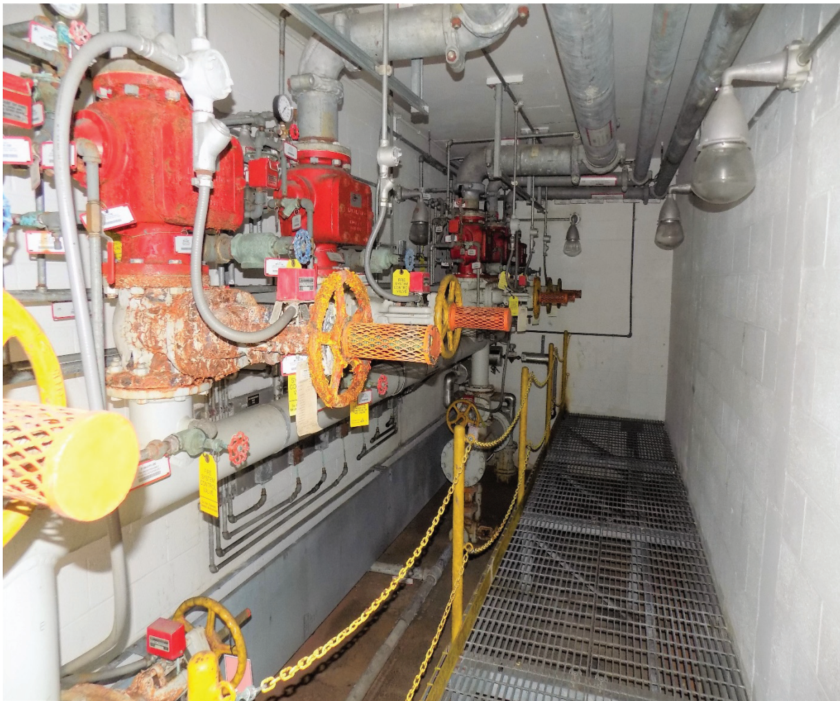
Figure 20. Building 484-9D, Valve Room (Looking East)
