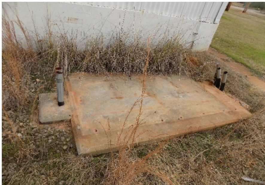
Figure 11. Building 483-3D, Old Location of Spill Control Motor Control Center
