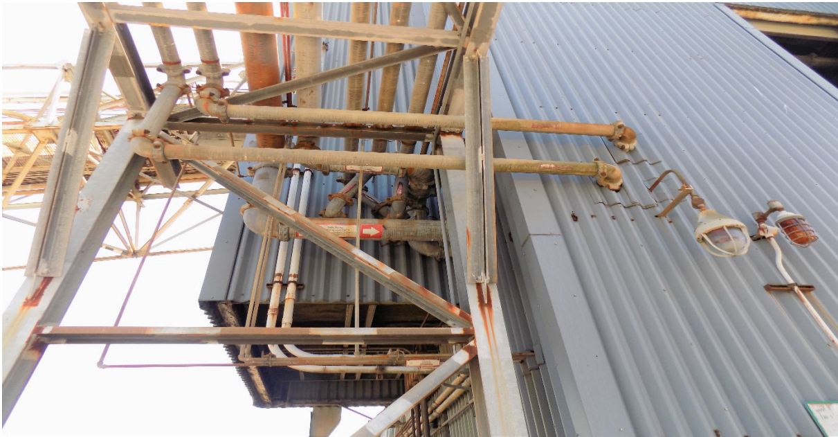
Figure 18. Pipe Bridge at the Coal Handling Crusher House (Looking Upward and South)
