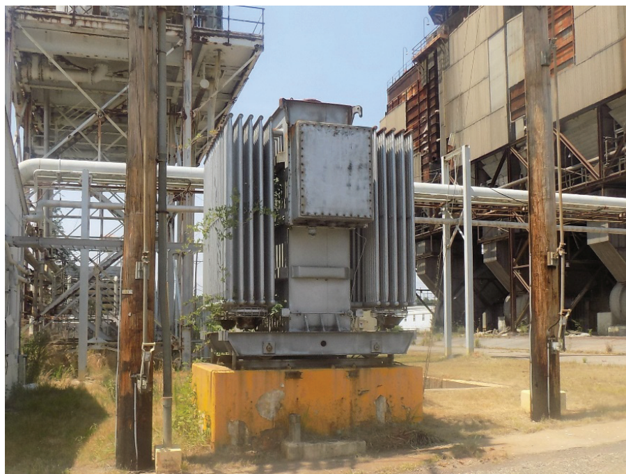
Figure 7. Transformer AT2W (Drained & Disconnected, outside scope of this SOW)
