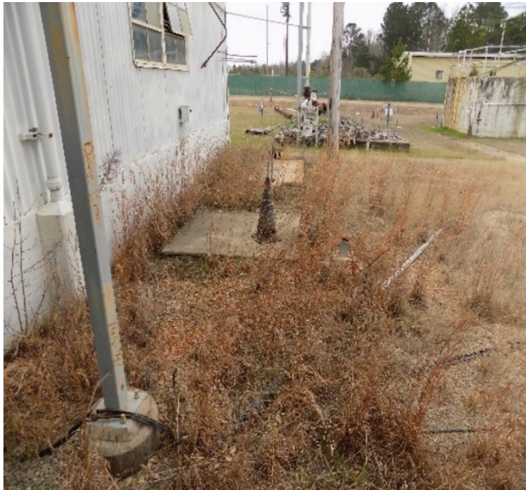
Figure 10. Building 483-3D, Old Location of Transformer W4
