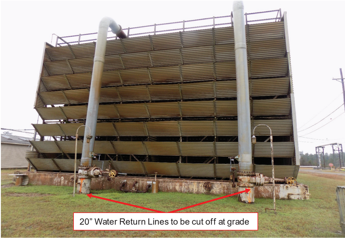
Figure 27. Building 485-D, D-Area Cooling Tower Water Return Lines
