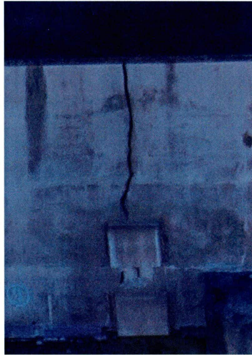
Figure 5: Crack on North Face
