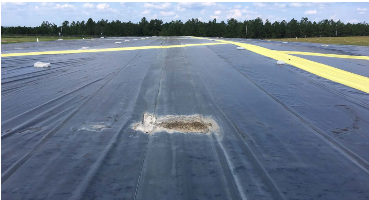
Figure F-8. Subsidence of Intact Covers (~1.5 m [5 ft] diameter) at Slit Trench Disposal Unit 5 (2016)
