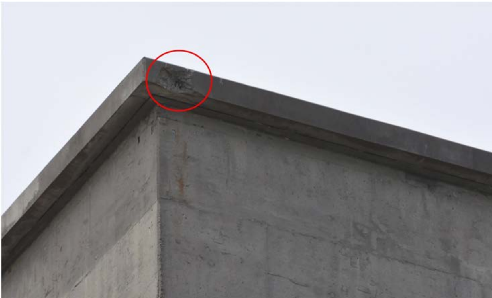
Figure N-6. View of 105-P Actuator Tower Roof Cap Flaw (2017)
