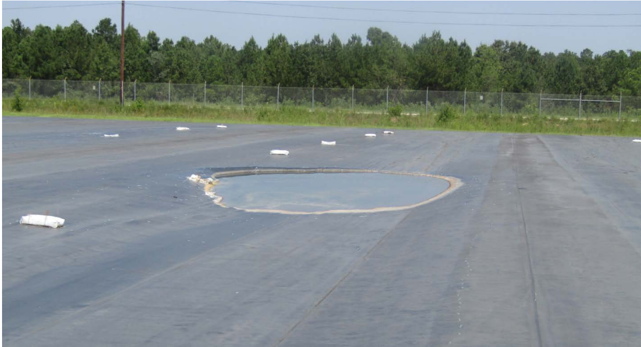
Figure F-7. Subsidence of Intact Covers (~3 m [10 ft] diameter) at Slit Trench Disposal Unit 4 (2016)
