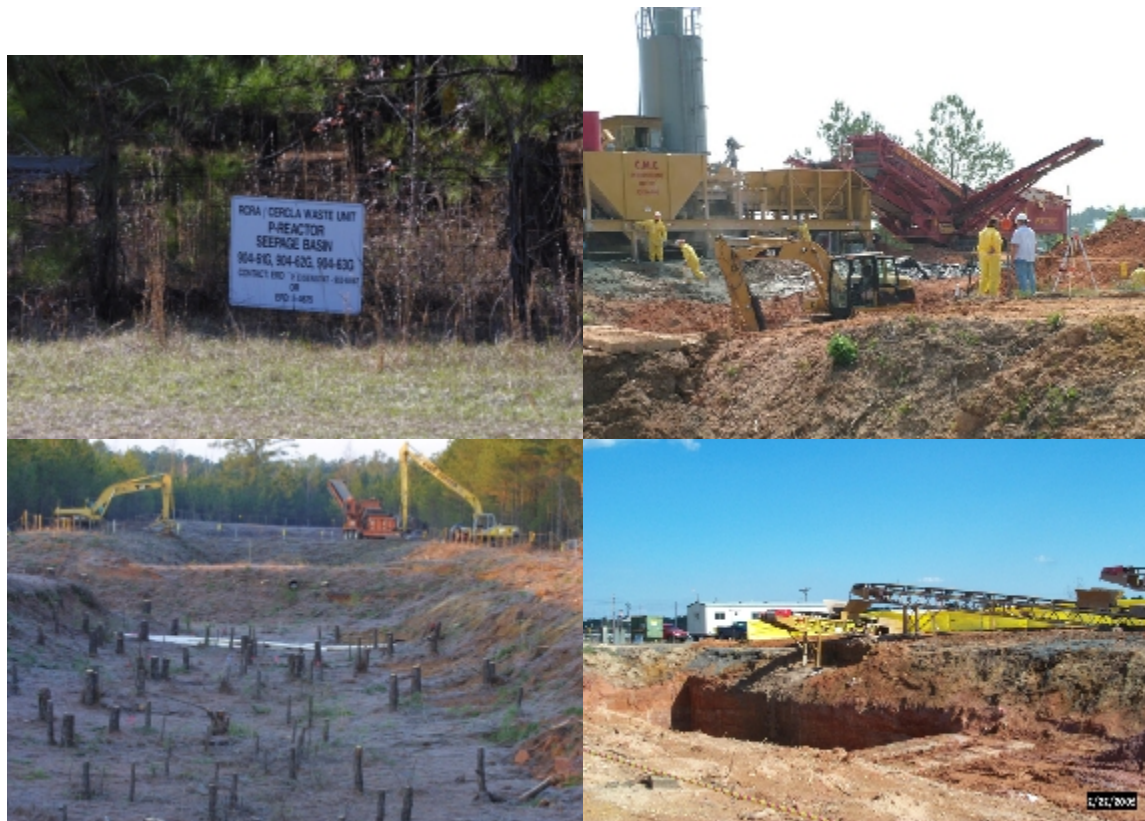
Figure O-3. Photographs from USDOE Archives Depicting the Remediation of the P- Reactor Seepage Basins (February 2004 through May 2005)
