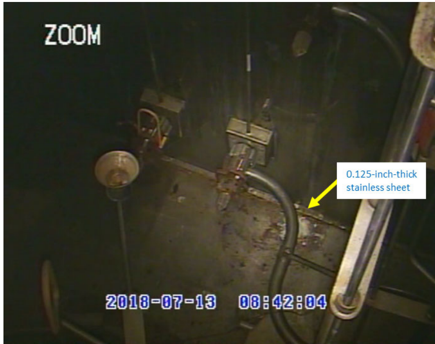
Figure 3: Accumulation of waste material Area A
