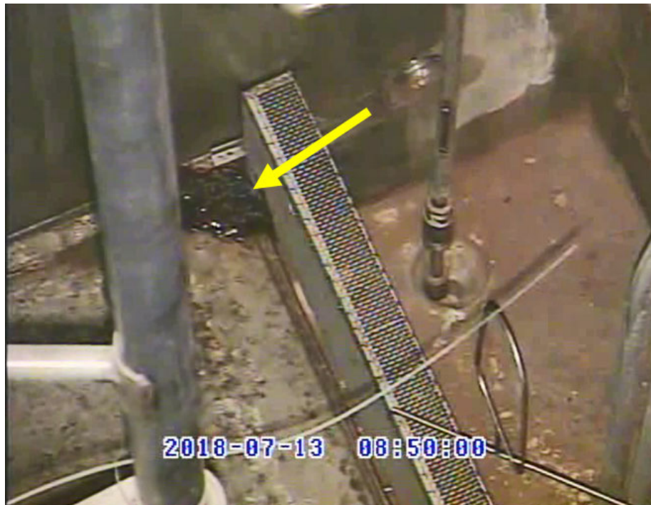
Figure 8: Foreign material on FDB-6 floor near sump Area D
