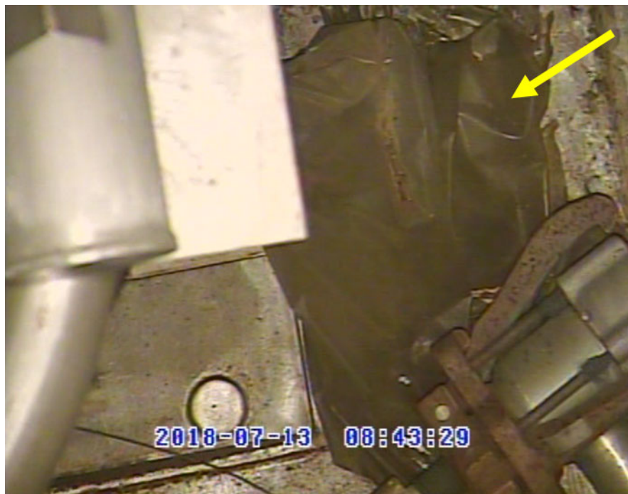
Figure 5: Foreign material on FDB-6 floor Area B
