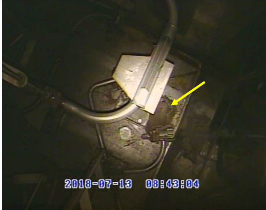
Figure 4: Foreign material on FDB-6 floor Area B
