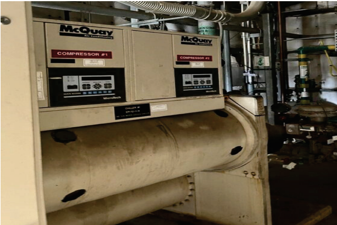
Photo 6 – Centrifugal Chiller (1 of 3)
