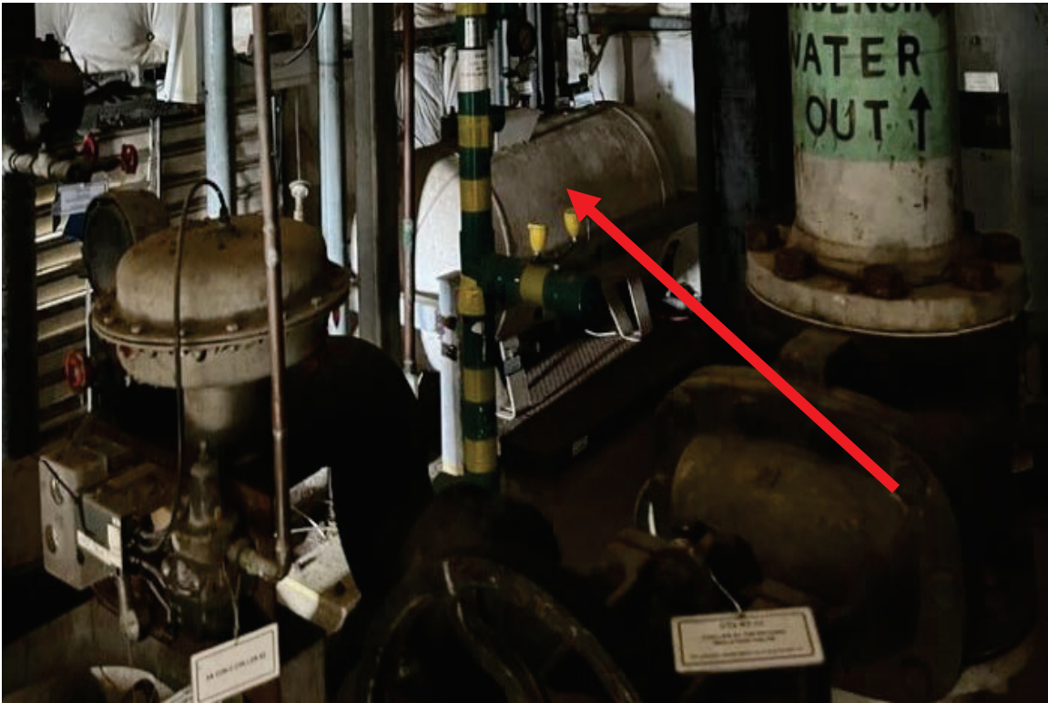
Photo 5 – Interior of Building 235-1F – Refrigerant Storage Tank
