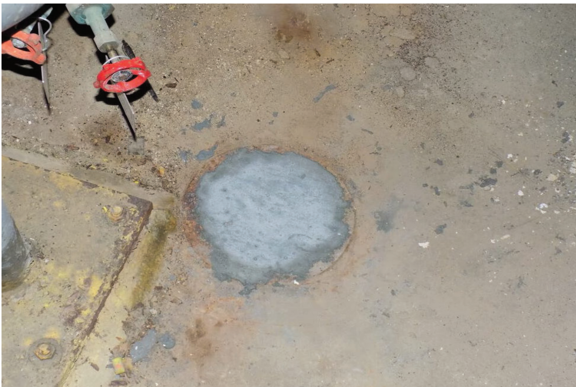
Photo 3 – Interior of Buildings 235-1F and 235-2F – Example of current state of drains.
