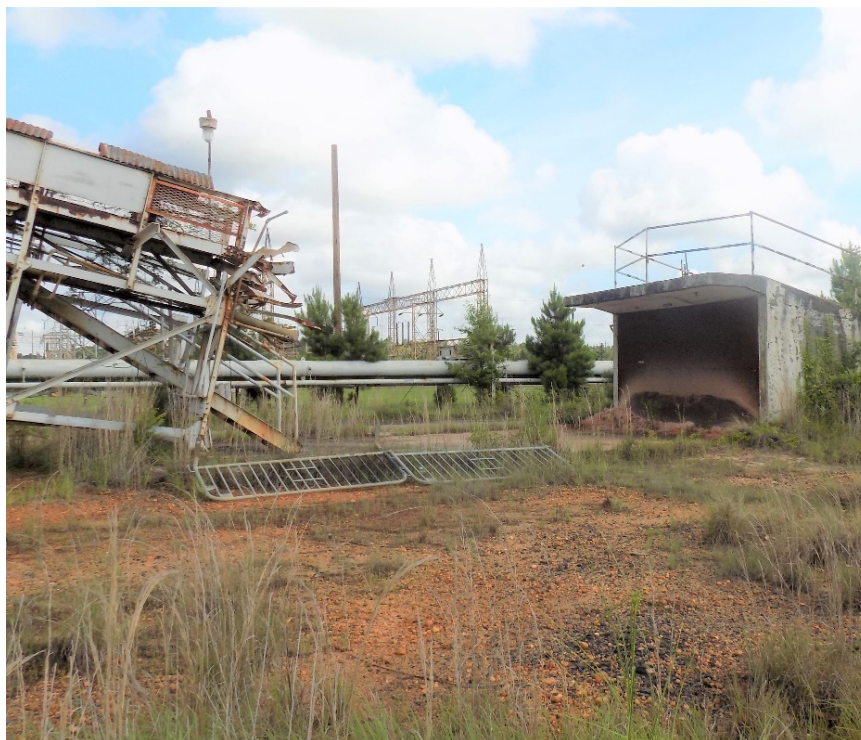
Figure 7. Photo of Conveyor No. 1 (cut) and Bunker Entrance to Conveyor No. 1 Tunnel
