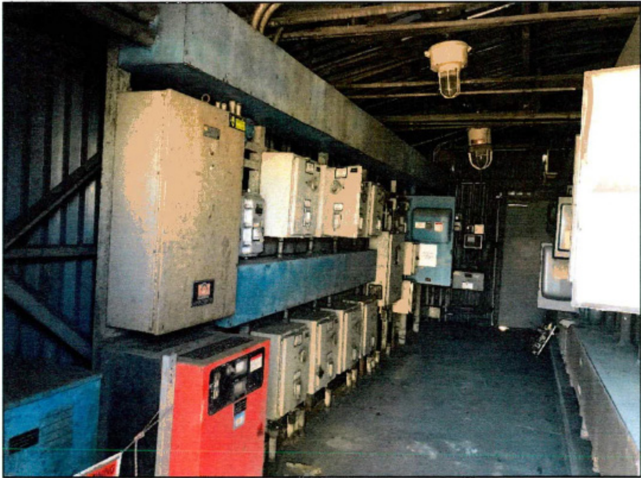
Figure 12. Inside the Coal Handling Control House
