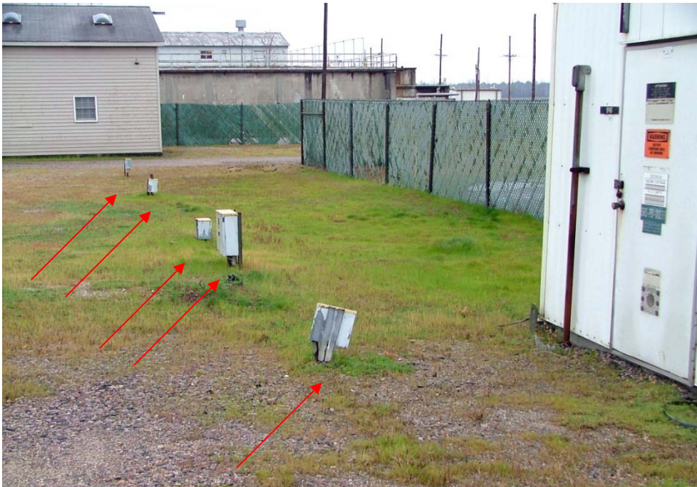
Figure 4. Building 704-7D, Exterior Electrical Feeder Boxes
