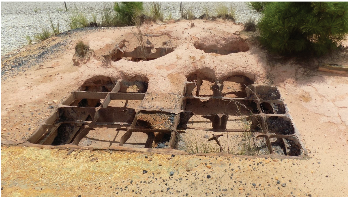
Figure A-16: Reclaim Hopper (Looking South) Before Decommissioning
