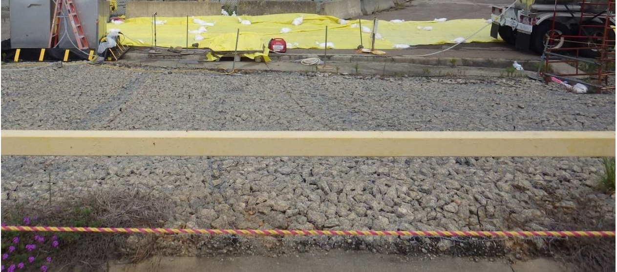
Above: Tuff tanks to culvert by rear of tanker (from left to right). Photo taken 7/5/22.
