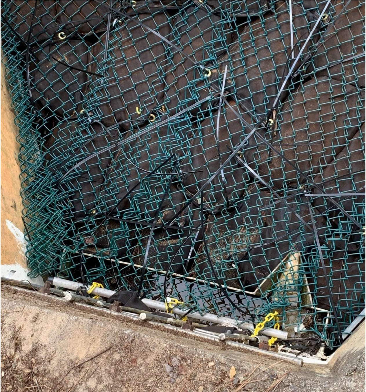
Above: Picture at H-06 Industrial Stormwater Outfall of secondary peat bed system installed with reinforcement on top of concrete. The primary peat bag section (not shown) is located inside and at the exit of the pipe leading to the outfall. The primary peat configuration is held in place by a rigid grate, therefore both the primary and secondary bag systems are supported. Photo taken on 7/9/22.
