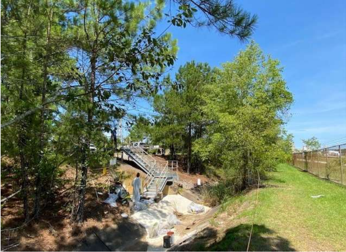
Above: Coating being applied to concrete at H-06 Industrial Stormwater Outfall on 7/7/22. Photo taken 7/7/22.
