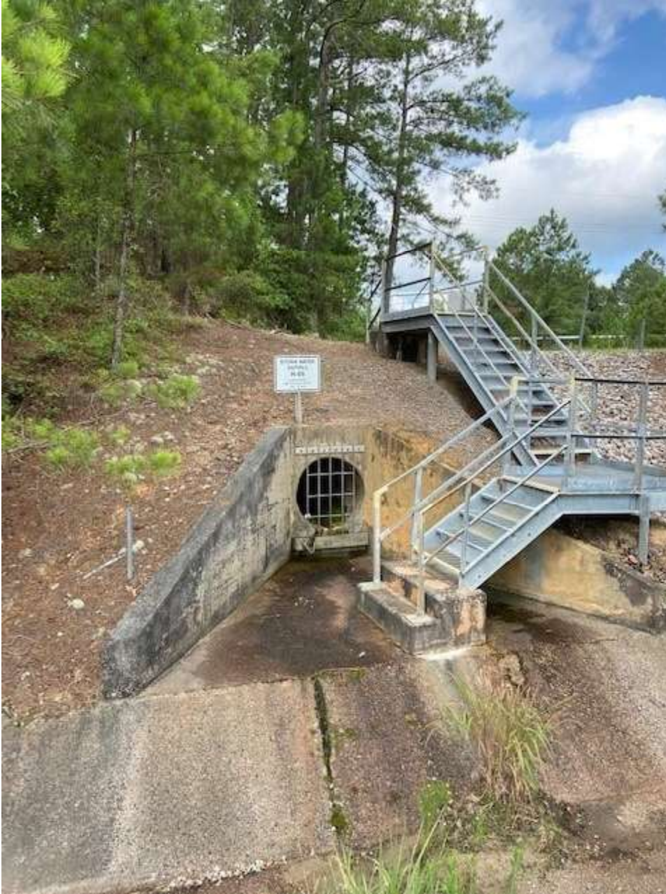
Above: Reinforced concrete pipe to H-06 Industrial Stormwater Outfall with damp paved area. Photo taken 7/5/22.
