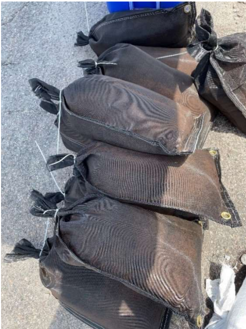
Below: Black permeable bags for filtration fabricated on site in response to spill. Installation of initial peat bags began on Thursday 7/7/22 followed by a controlled flush of the pipe leading to the outfall. Photo taken on 7/8/22.
