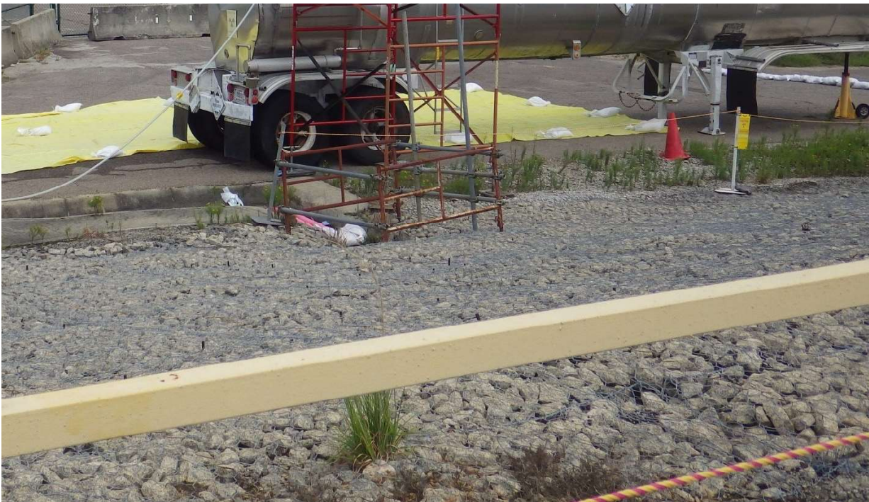
Below: Rear of tanker and culvert to reinforced concrete pipe. Photo taken 7/5/22.
