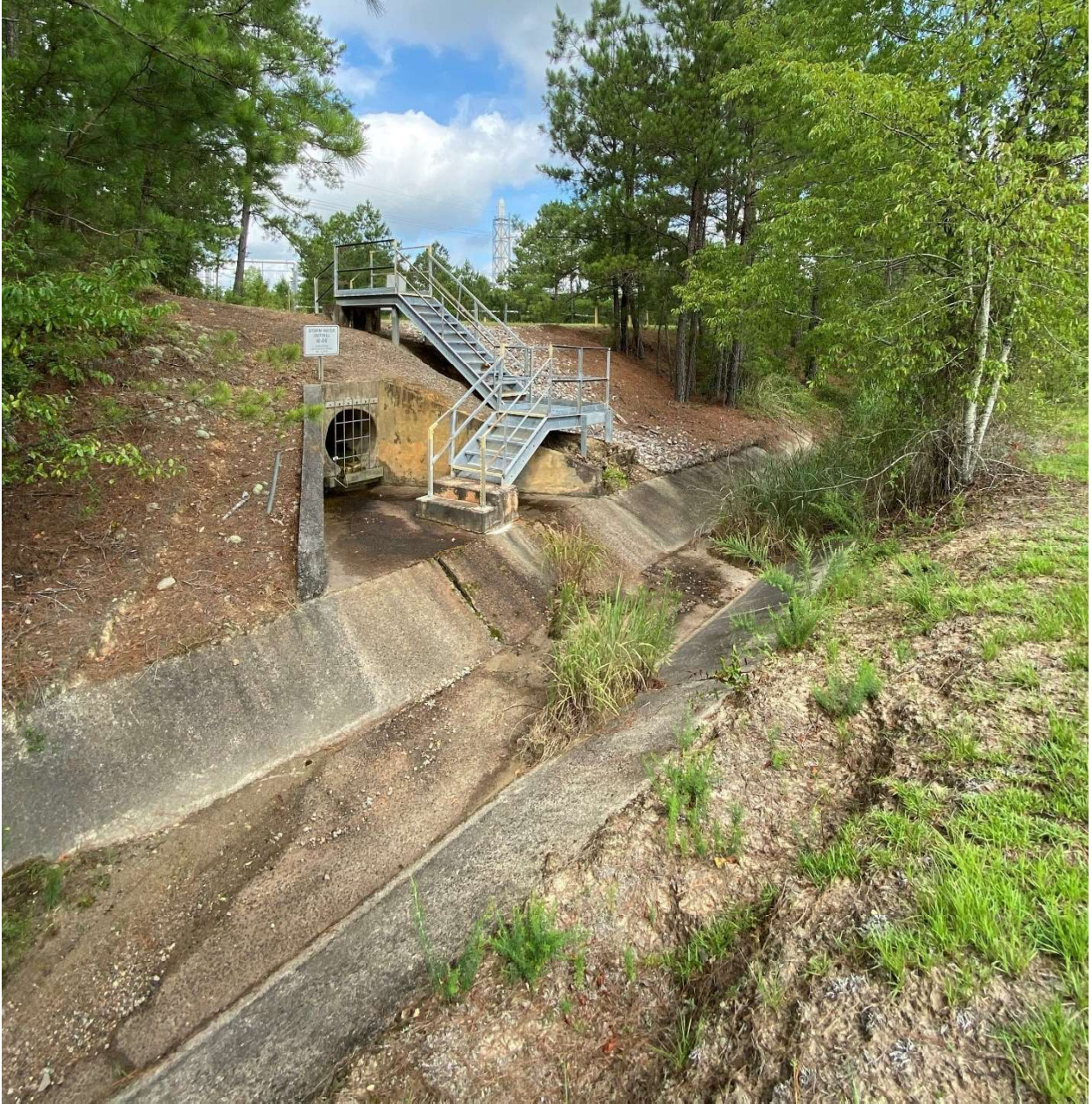
Above: H-06 Industrial Stormwater Outfall looking upstream of concrete ditch. Photo taken 7/5/22.
