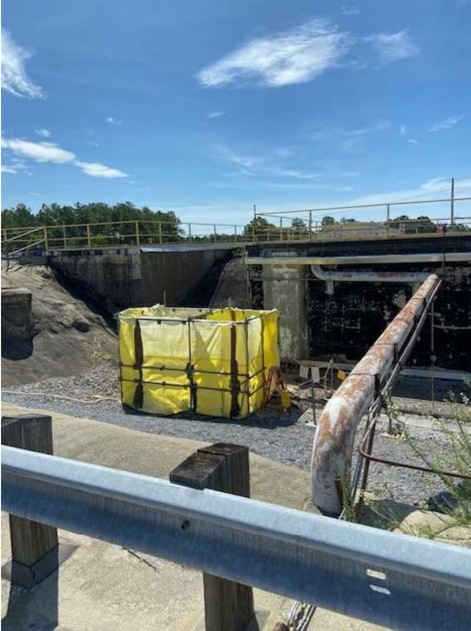
Above: Sand Filter sump location that pumps to tuff tanks. Photo taken 7/5/22.
