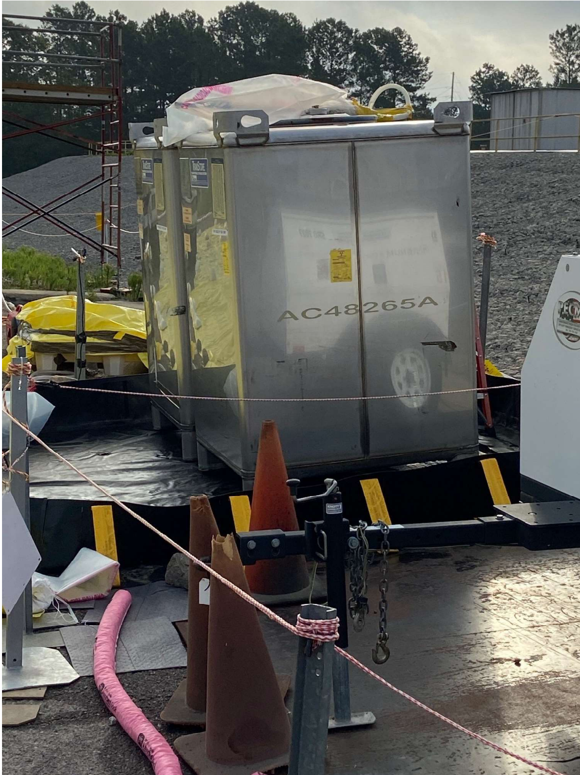
Above: Two tuff tanks (550 gallons each, one empty prior to spill). Temporary dike installed around tanks prior to spill. Photo taken 7/5/22.
