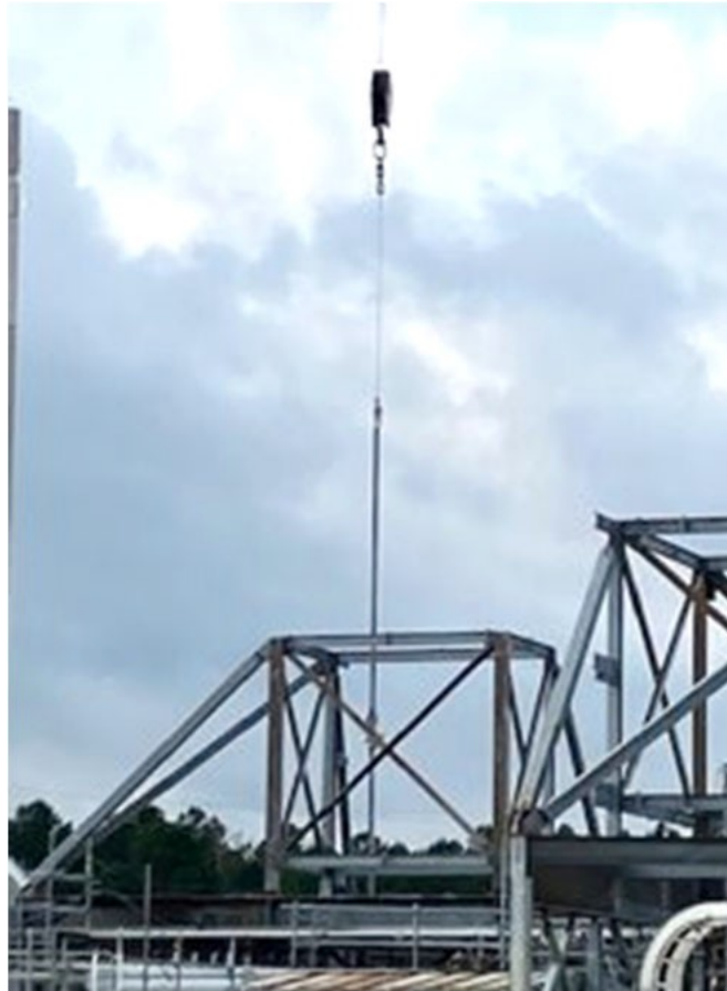
Figure 12 - Tank 28F Riser B3 Low Volume Mixing Jet
