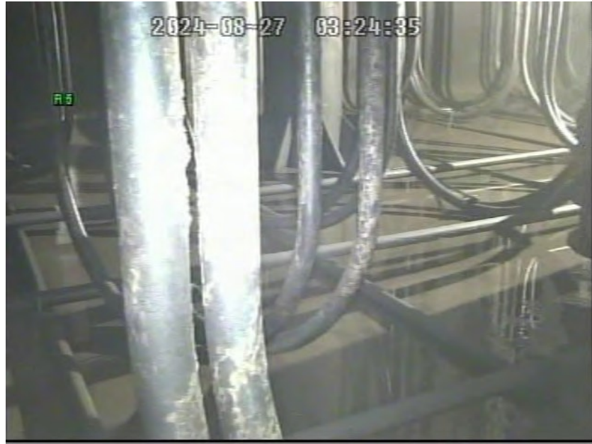
Figure 3 - Tank 9H Primary Tank (Post-Waste Removal)
