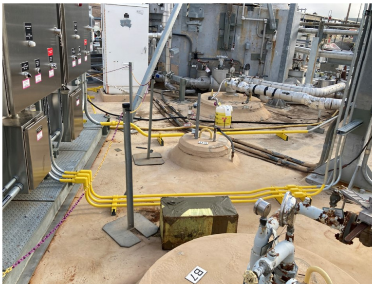
Figure 13 - Tank 31H Gas Release Mode Skid Conduit
