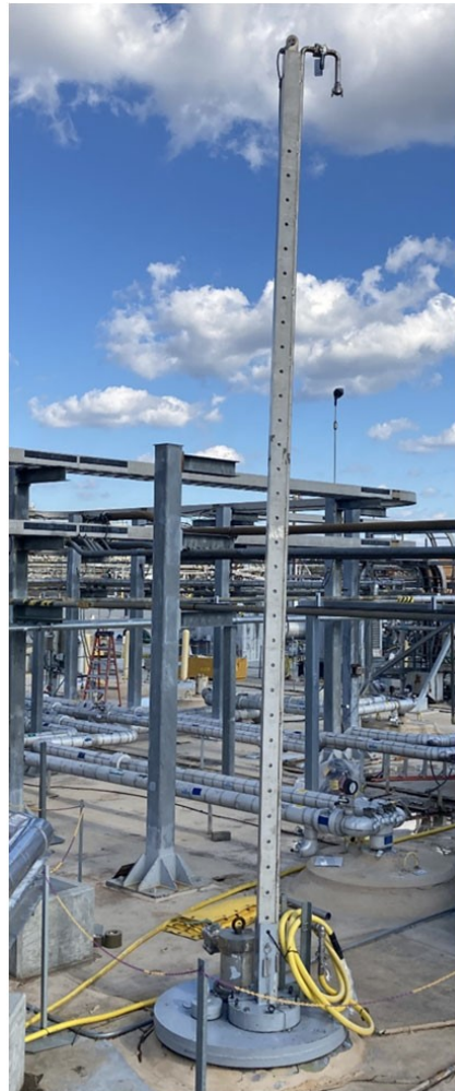
Figure 15 - Tank 31H Riser H Low Volume Mixing Jet
