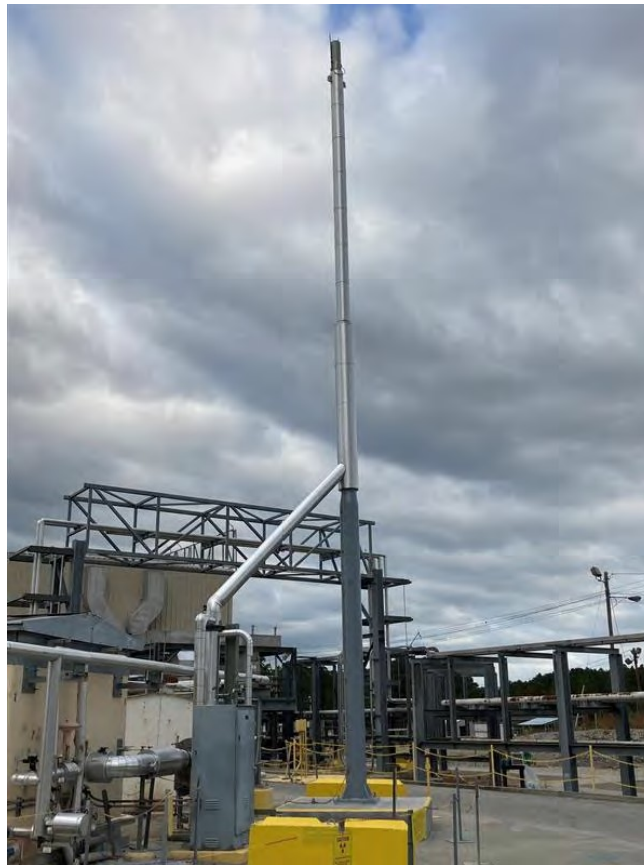
Figure 20 - Tank 47F Heating and Ventilation
