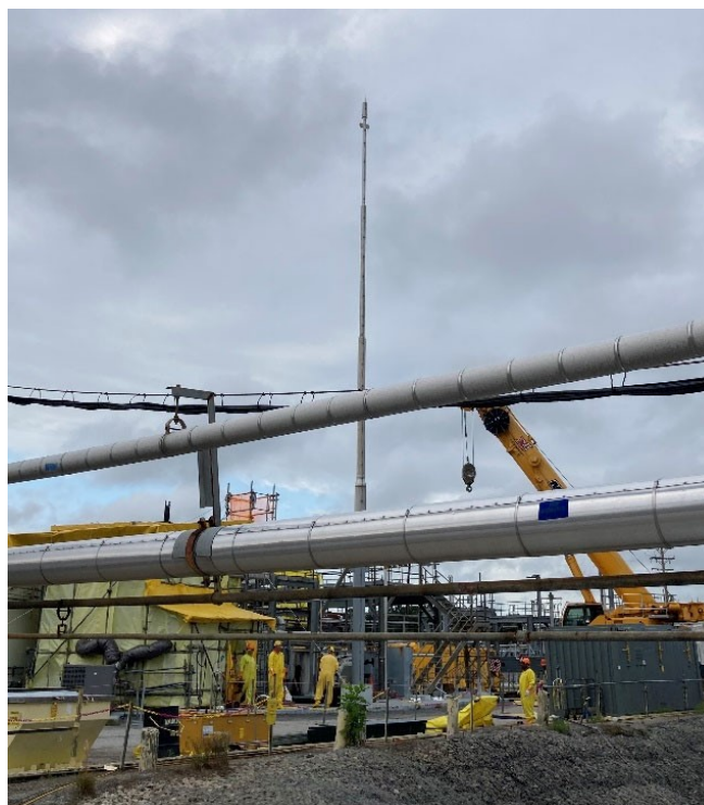
Figure 8 - Tank 14H H&V Purge Stack Extension
