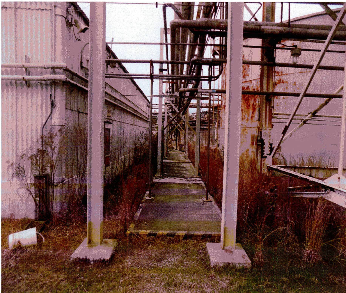
Figure 7. Building 483-3D Cable Trench
