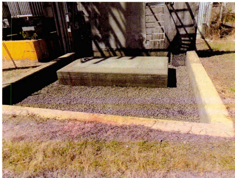
Figure 6. Transformer AT1W Transformer Pad Location with Containment Dike
