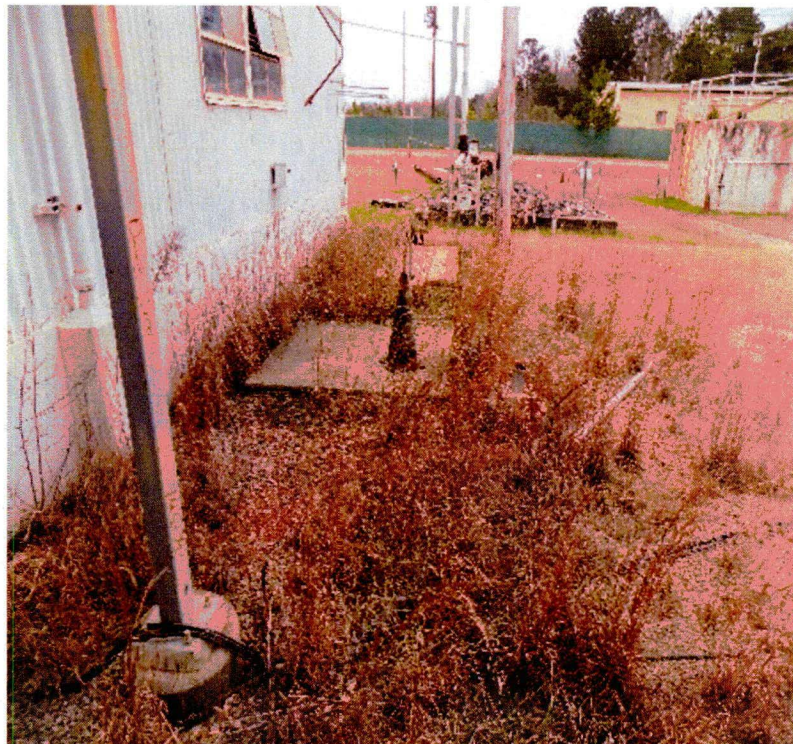
Figure 8. Old Location of Transformer W4
