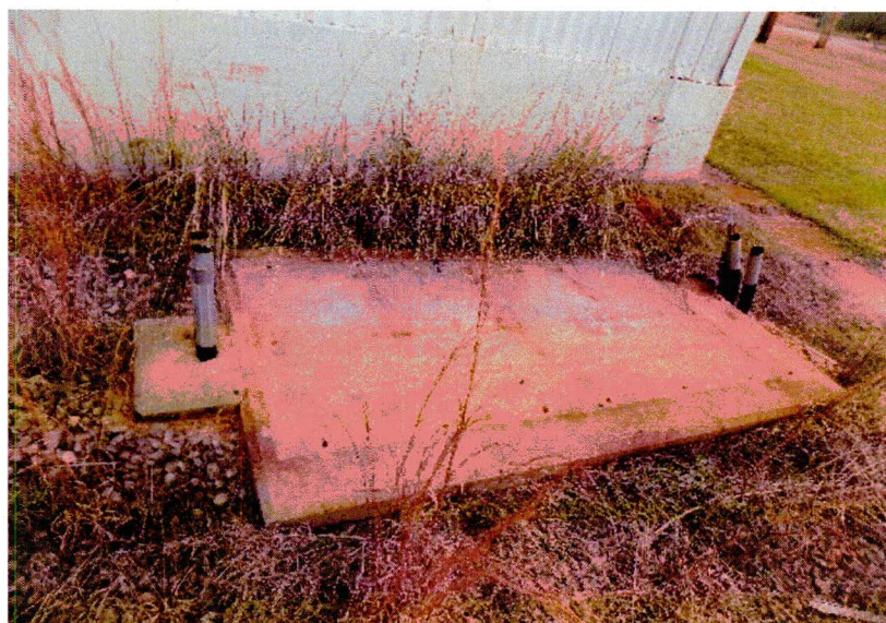
Figure 9. Old Location of Spill Control Motor Control Center
