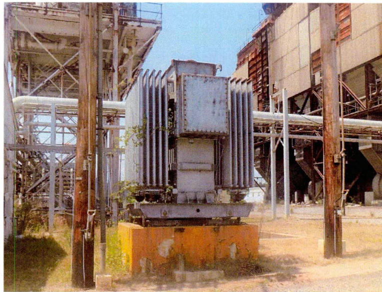
Figure 5. Transformer AT2W (Drained & Disconnected)
