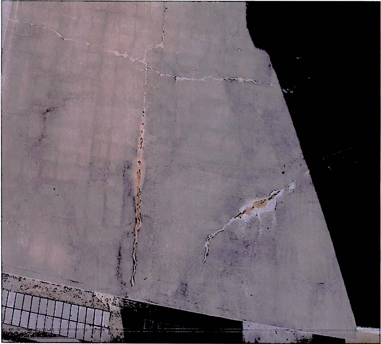
Cracking on Roof, North of High-hat
