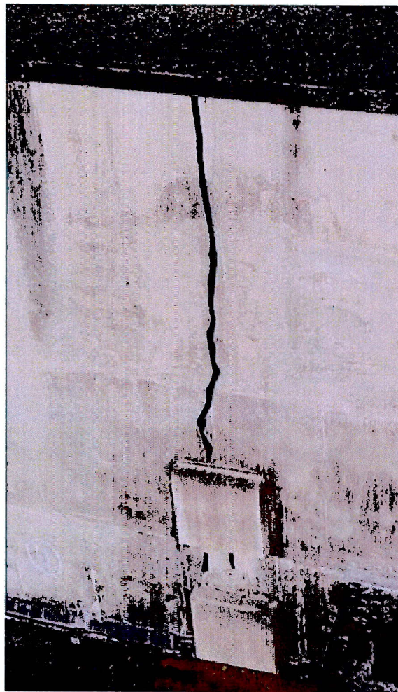
Crack, North Face
