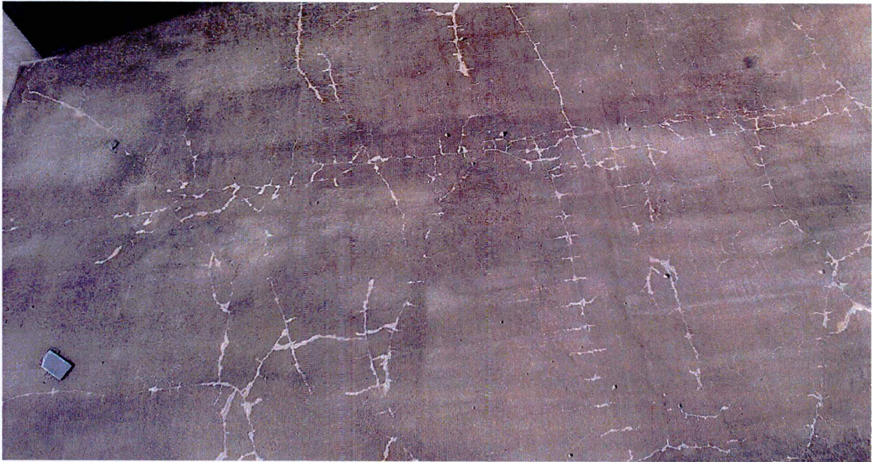
Cracking and Minor Spalding, Gantry Crane Roof
