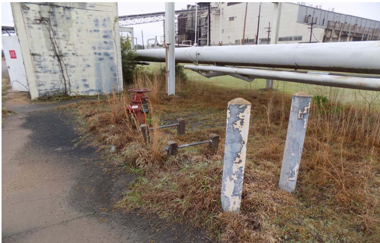
Figure 8. Building 484-9D Hydrant, Support Frame and Bollards
