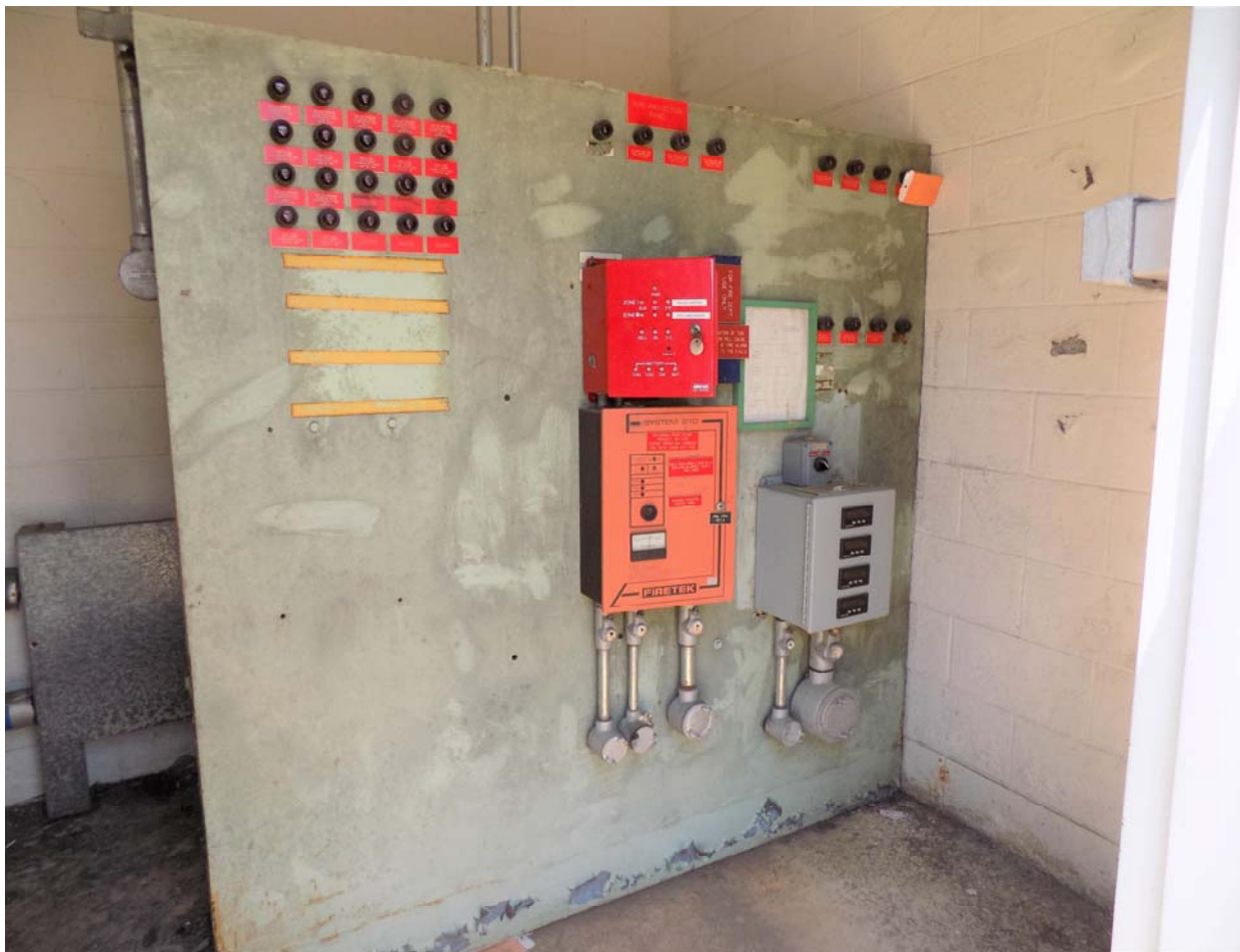
Figure 7. Fire Panel and Control Room (Looking Northeast)
