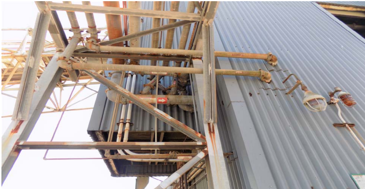
Figure 3. Pipe Bridge at the Coal Handling Crusher House (Looking Upward and South)
