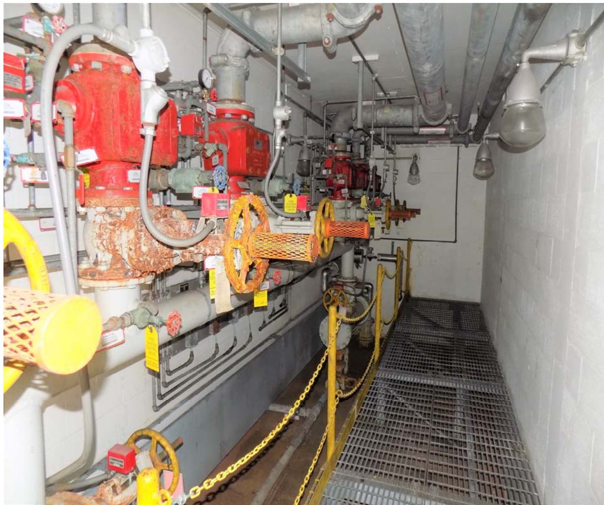
Figure 6. 484-9D Valve Room (Looking East)
