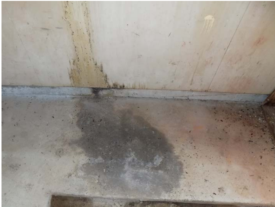
Figure 3. Stain in Storage 8
