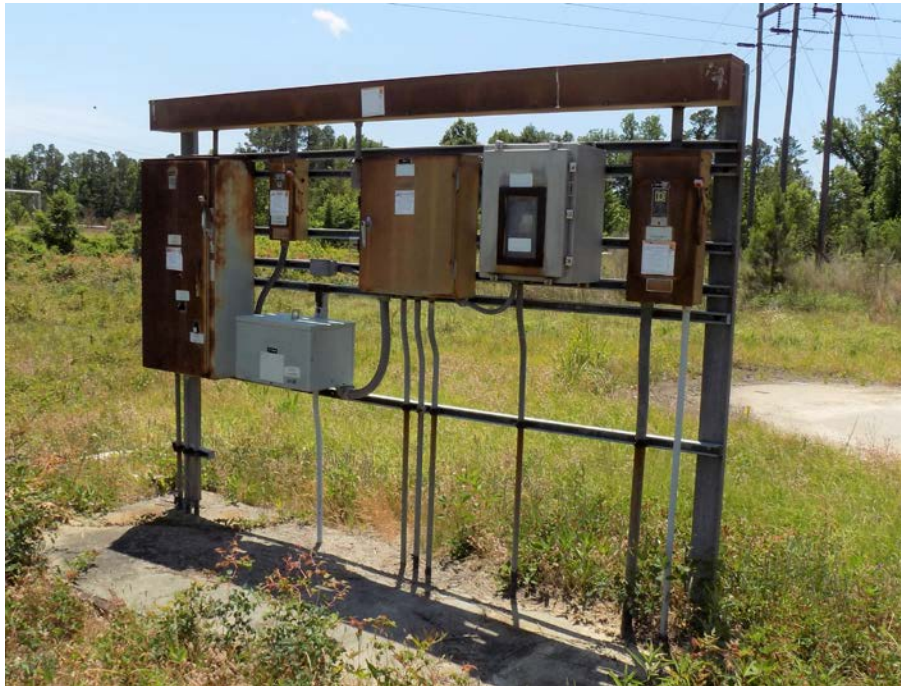
Figure 11. 905-3D Primary Domestic Well Electrical Panel
