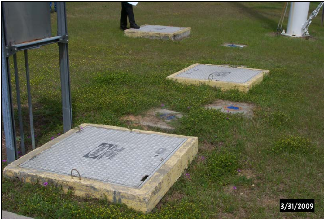
Figure 17. Domestic Water Facility Clear Well Check Valve and Water Meter Structures (Near) and Chlorine Injector Structure (Far)
