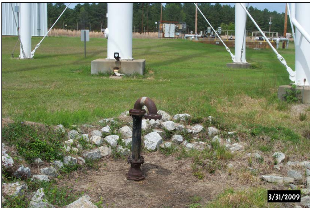
Figure 14. Building 905-5D Elevated Domestic Water Storage Tank Drain
