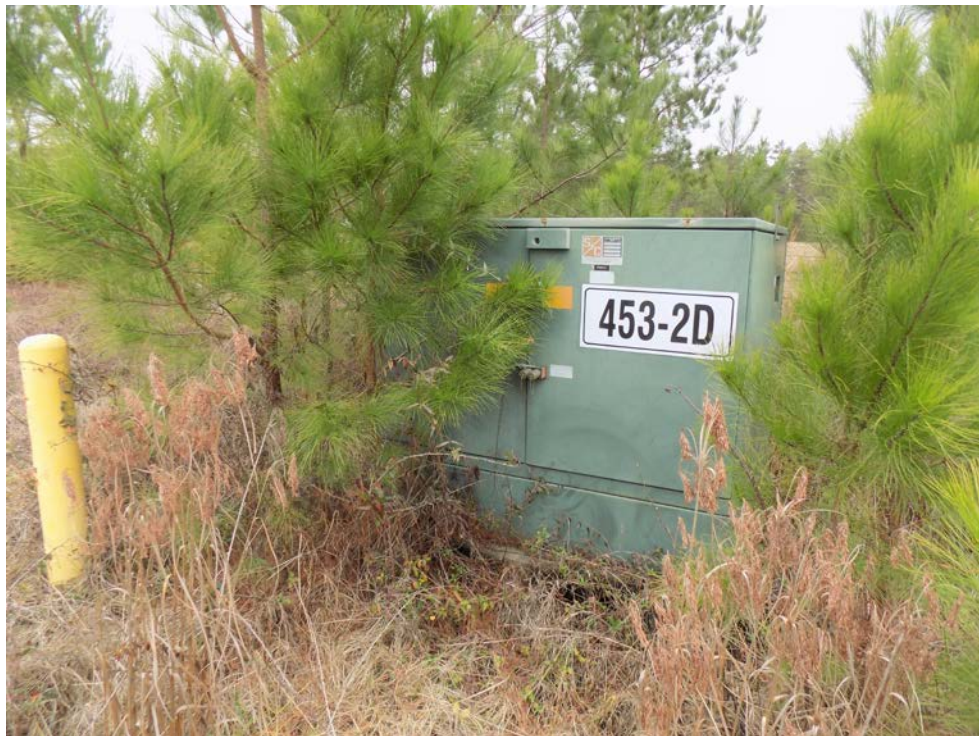
Figure 19. 453-2D - Air Switch AS-1
