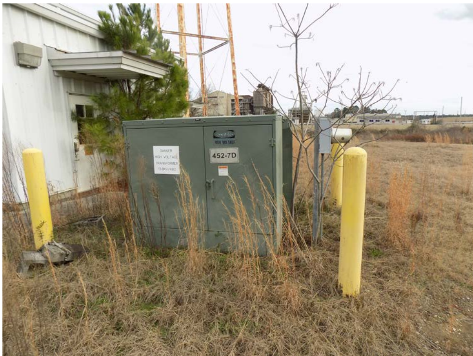
Figure 20. 452-7D, Transformer (T-1) for Domestic Water System
