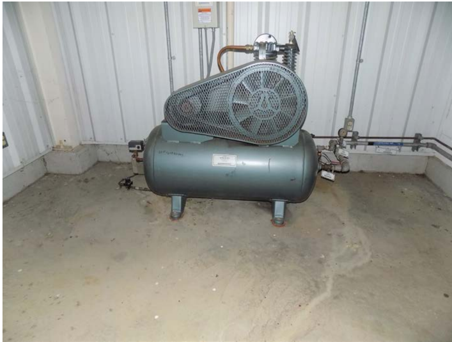
Figure 5. Building 483-7D Instrument Air Compressor
