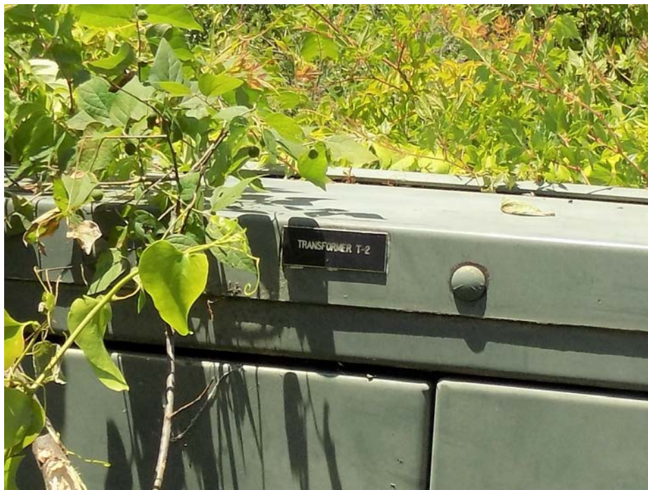
Figure 22. 452-11D, Transformer (T-2) for Domestic Water System
