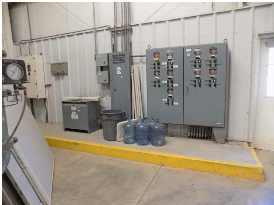
Figure 4. Building 483-7D Electrical Control Pad
