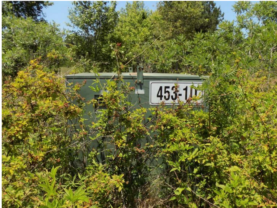
Figure 21. 453-1D, Air Switch AS-2
