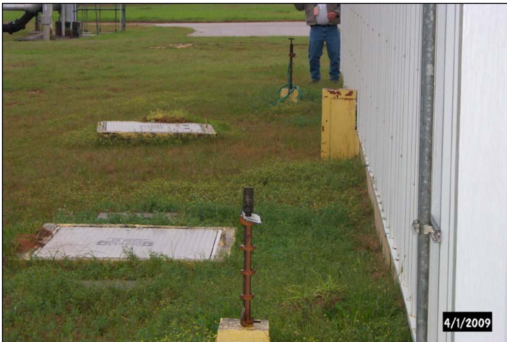
Figure 18. Incoming Domestic Water Meter Pit (Near Left) and Polyphosphate Injection Structure (Far Left) and Yard Hydrants
