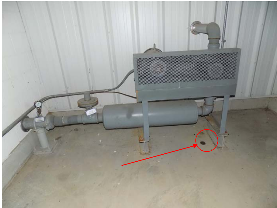
Figure 6. Building 483-7D Backwash Air Scour Blower
