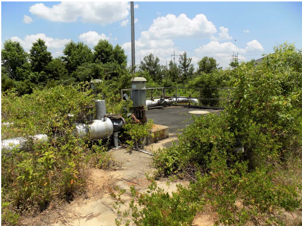
Figure 15. Domestic Water Facility Clear Well
