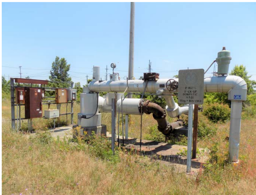
Figure 12. 905-136D Back-Up Domestic Well & Electrical Panel
