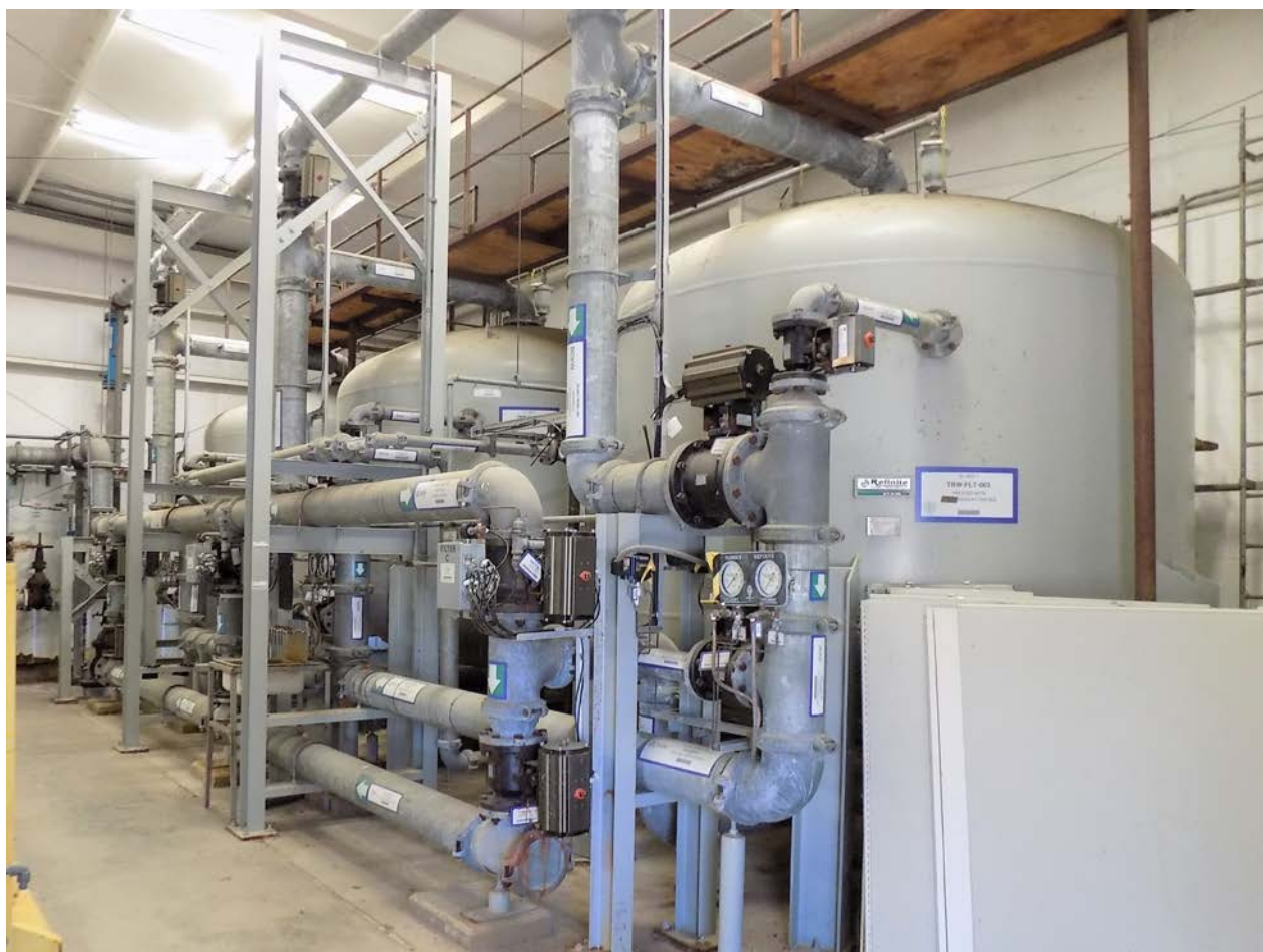
Figure 7. Building 483-7D Sand Filters
