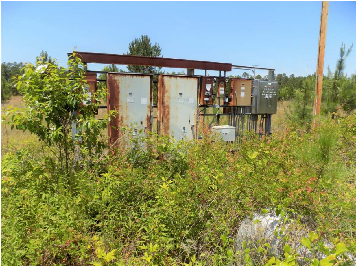
Figure 16. Domestic Water Facility Clear Well Electrical Panel
