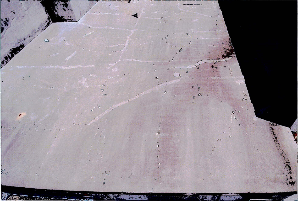
Cracking, Gantry Crane Roof
