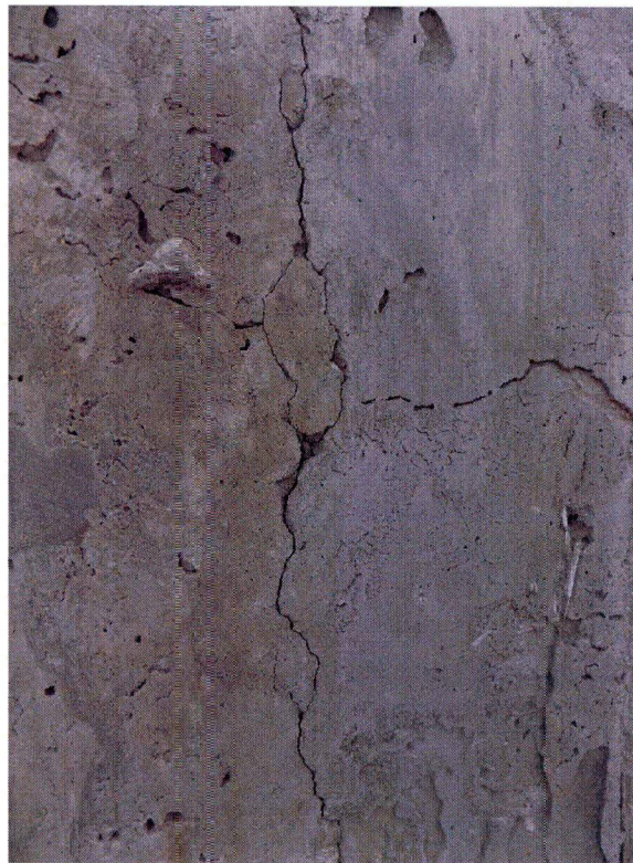
Cracking, 105-R Concrete – Dissassembly Side
